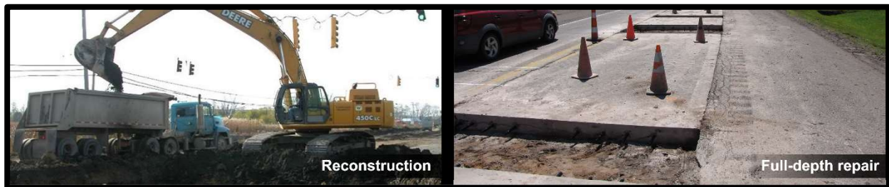
Figure 2: Examples of reconstruction treatments—(left) reconstructing a road and (right) road prepared for full-depth repair.
