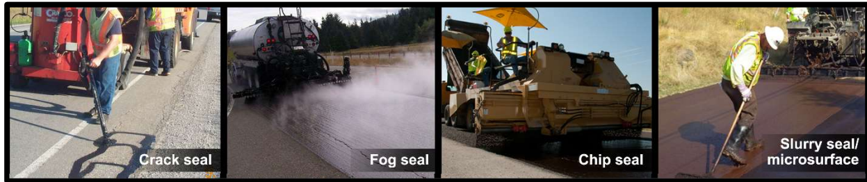
Figure 4: Examples of capital preventive maintenance treatments—(from left) crack seal, fog seal, chip seal, and slurry seal/microsurface.
