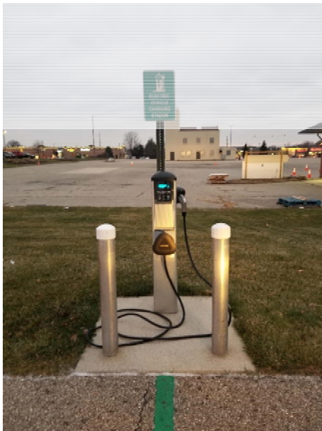
Level 3 Charging Station at Family Fare Quick Stop
