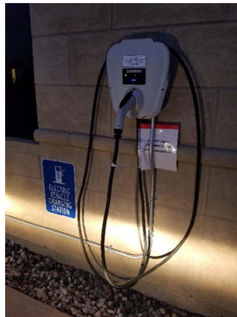
Level 2 Charging Station at Gastrointestinal Associates of Western Michigan
