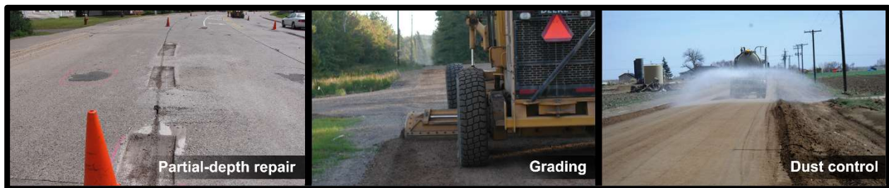
Figure 5: Examples of capital preventive maintenance treatments, cont'd—(from left) concrete road prepared for partial-depth repair, gravel road undergoing maintenance grading, and gravel road receiving dust control application (dust control photo courtesy of Weld County, Colora, weldgov.com).
