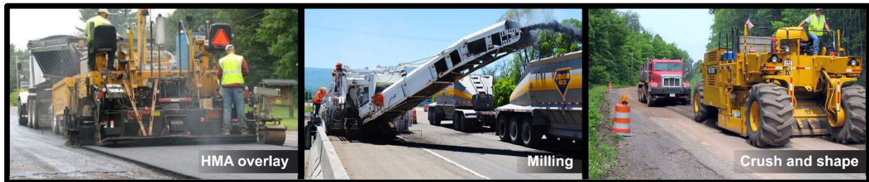
Figure 3: Examples of structural improvement treatments—(from left) HMA overlay on an unmilled pavement, milling asphalt pavement, and pulverization of a road during a crush-and-shape project.
