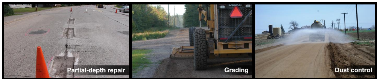
Figure 5: Examples of capital preventive maintenance treatments, cont'd—(from left) concrete road prepared for partial-depth repair, gravel road undergoing maintenance grading, and gravel road receiving dust control application (dust control photo courtesy of Weld County, Colorado, weldgov.com).
