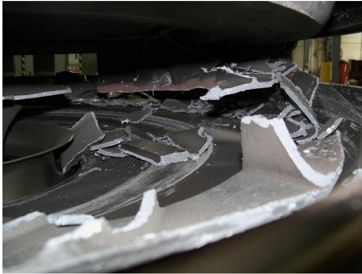
Blower Failure Picture 2
