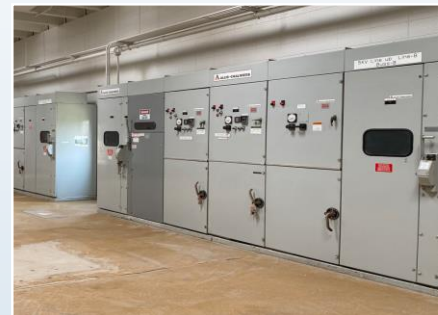
A Electrical Distribution
