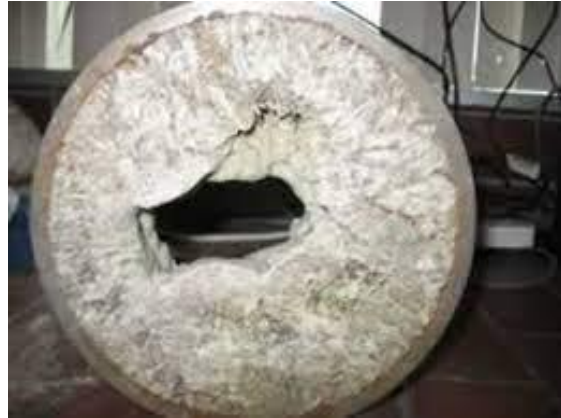
Figure 4: Struvite formation in a pipe
