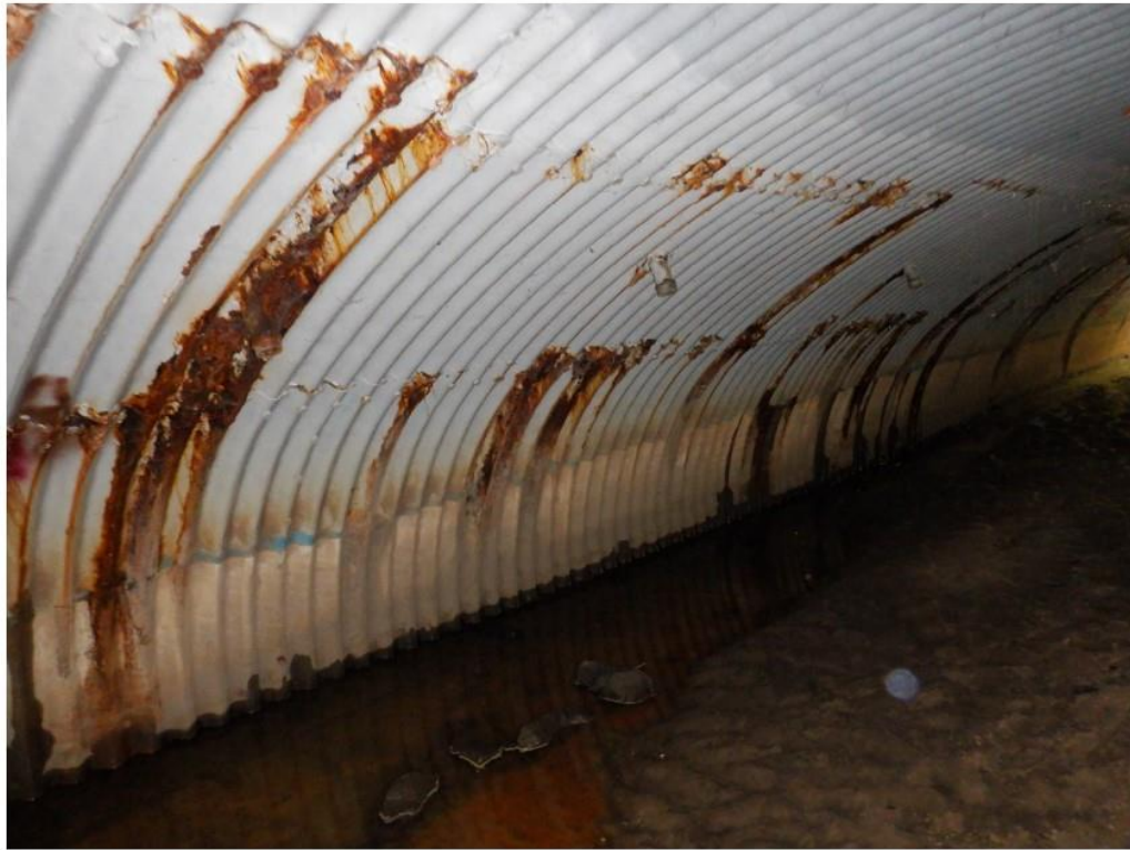
AREAS OF HEAVY CORROSION ON WEST WALL OF EAST BARREL
