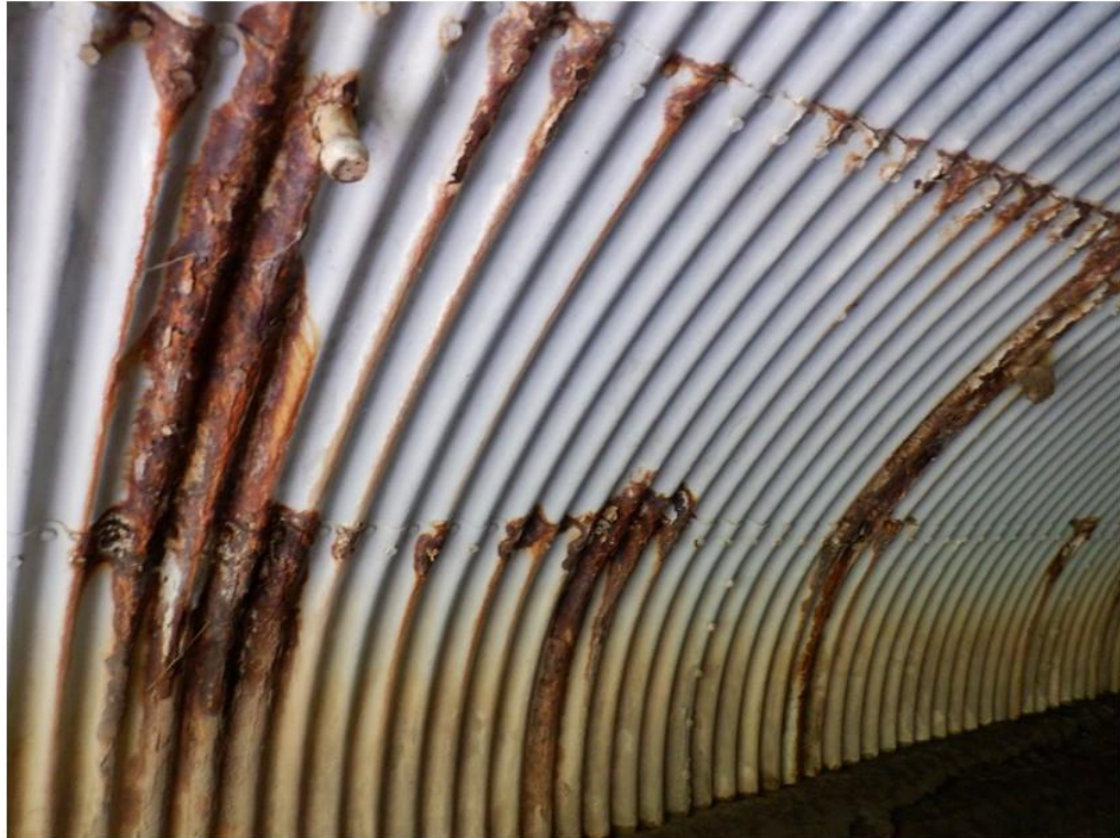
HEAVY CORROSION ON EAST WALL OF WEST BARREL
