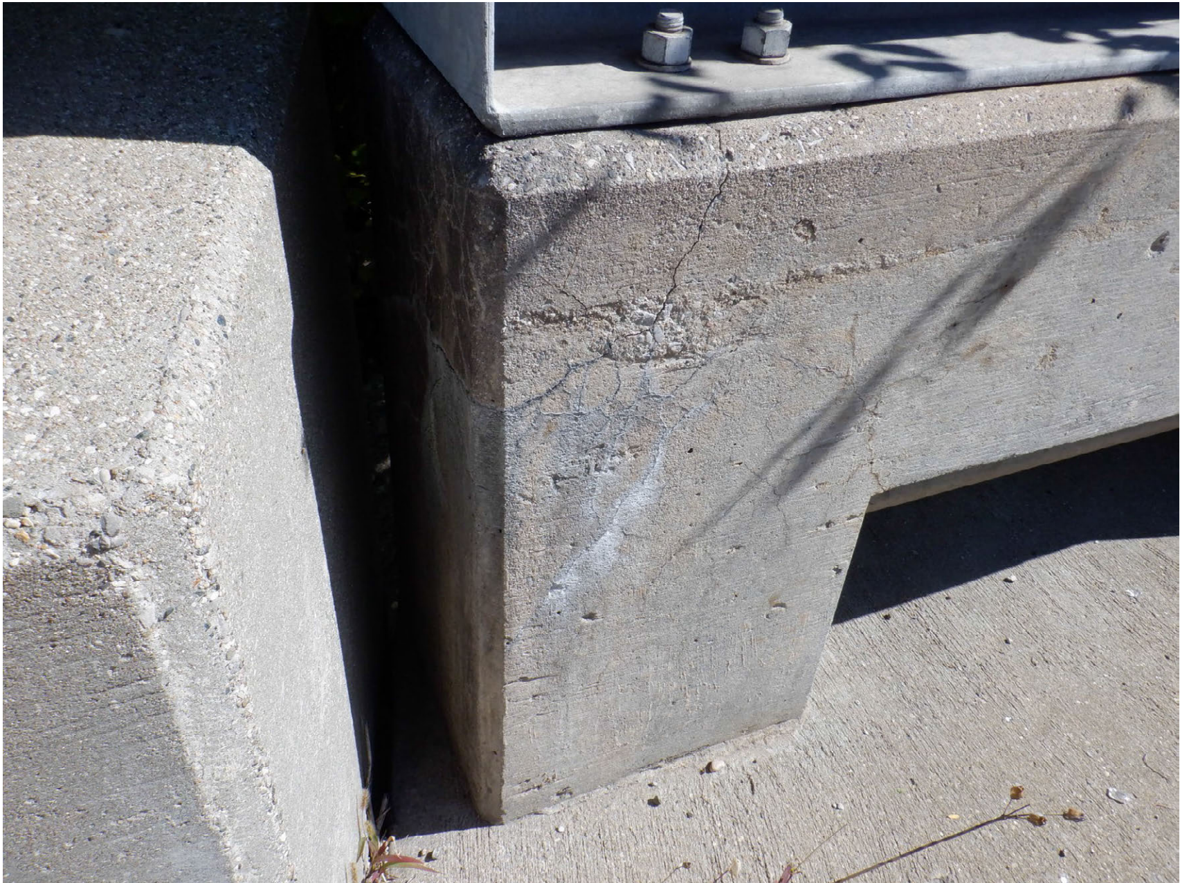
MAP CRACKING AT NORTH END OF EAST PARAPET
