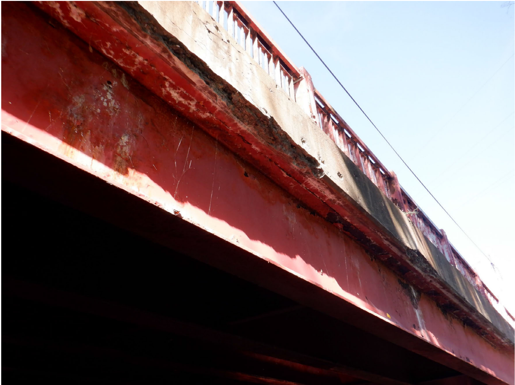
SPALLING ON BOTTOM OF EAST DECK FASCIA
