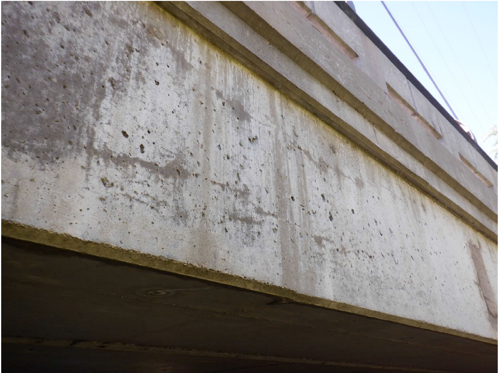
HAIRLINE CRACKING IN EAST FASCIA
