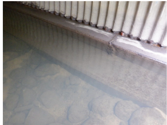
Exposed footing in west barrel
