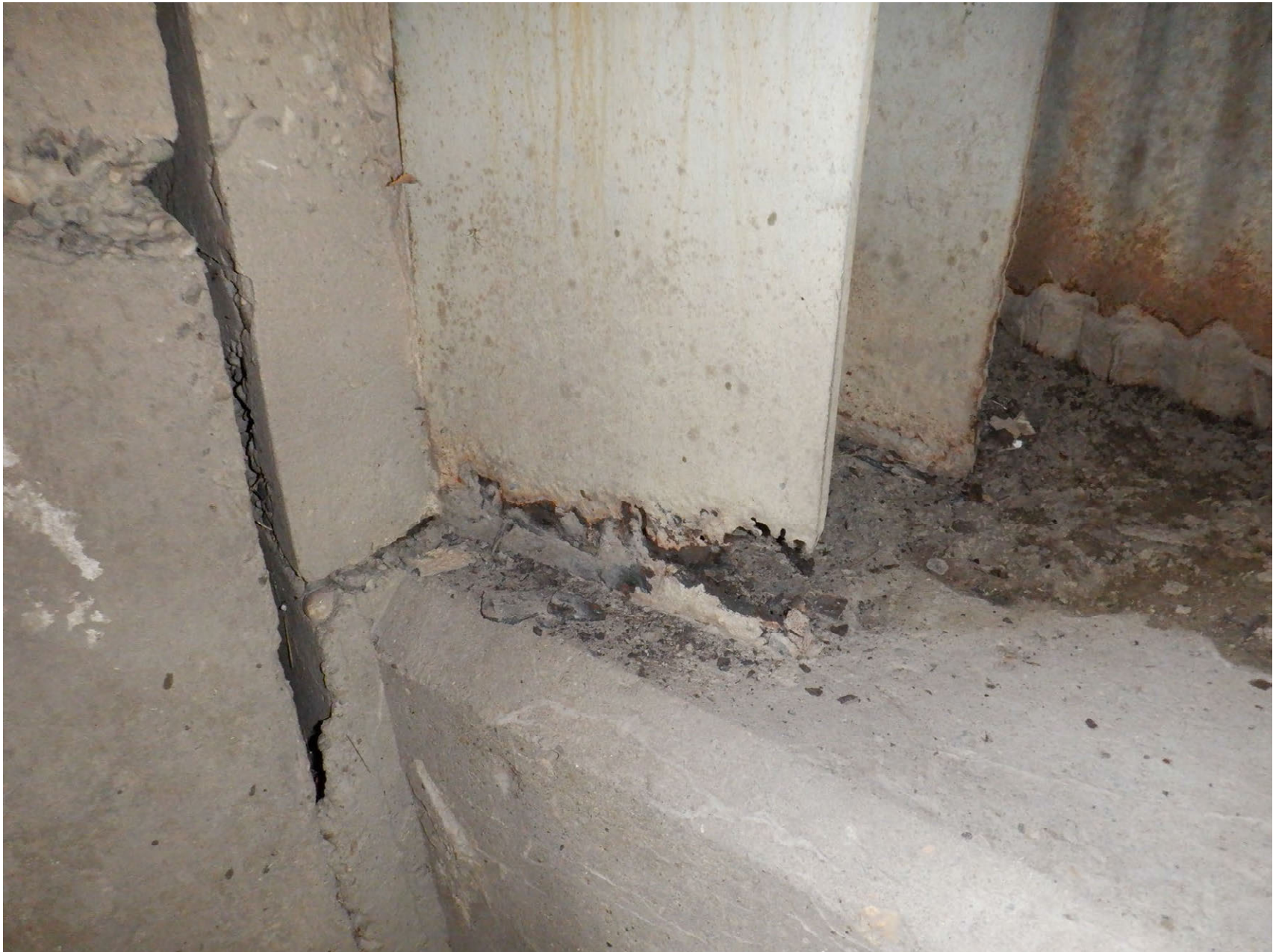
HOLE AT BOTTOM OF NORTH ABUTMENT PILE UNDER WEST FASCIA
