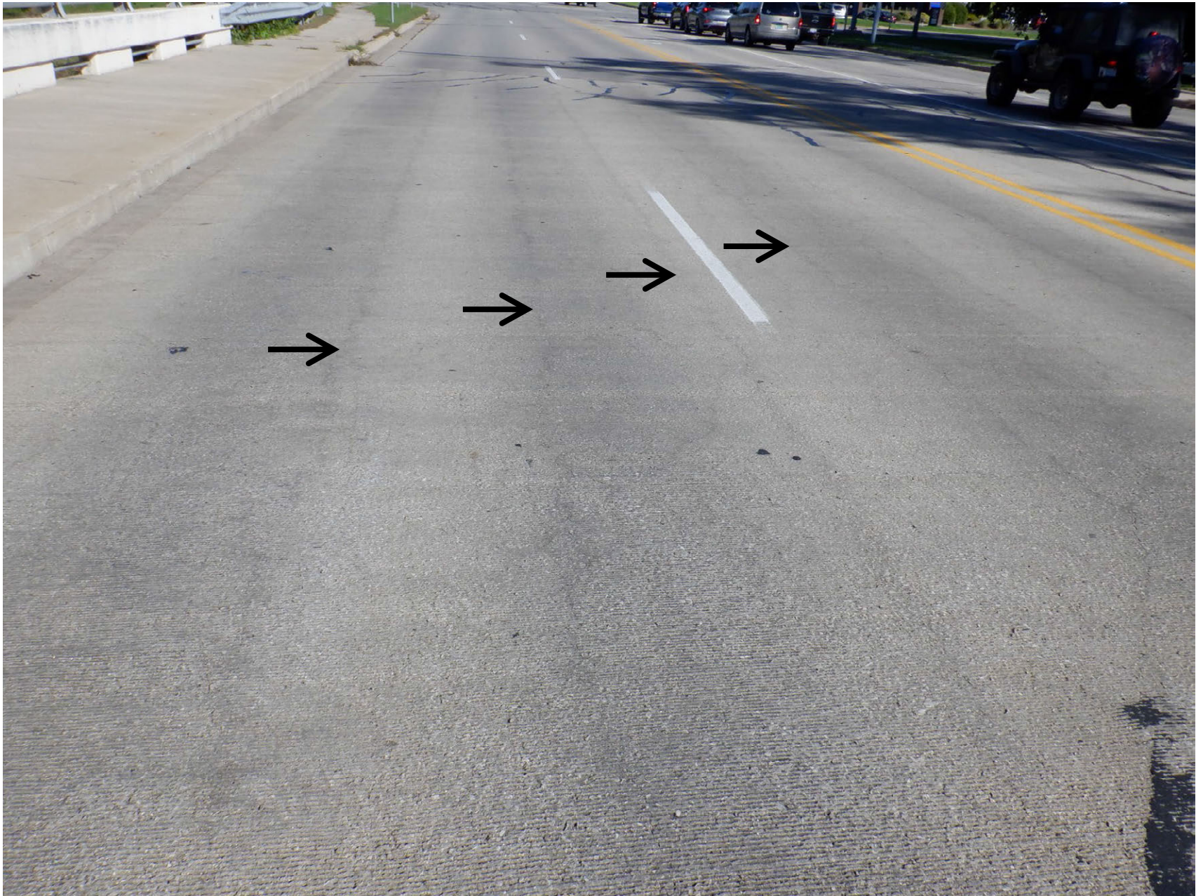
HAIRLINE CRACKS IN CONCRETE DECK SURFACE ALONG BEAM LINES
