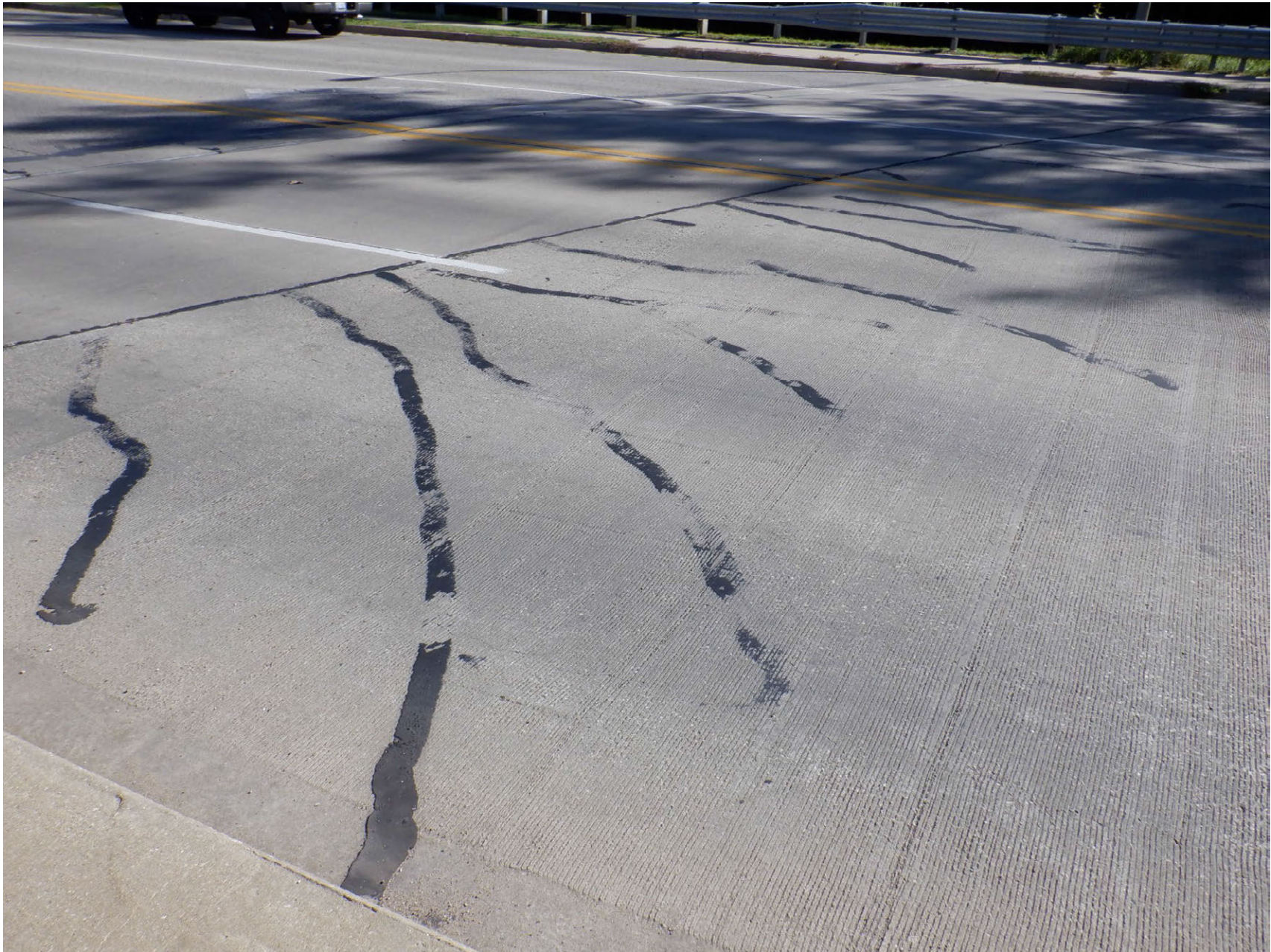
PREVIOUSLY SEALED CRACKS IN CONCRETE DECK SURFACE PERPENDICULAR TO NORTH REFERENCE LINE
