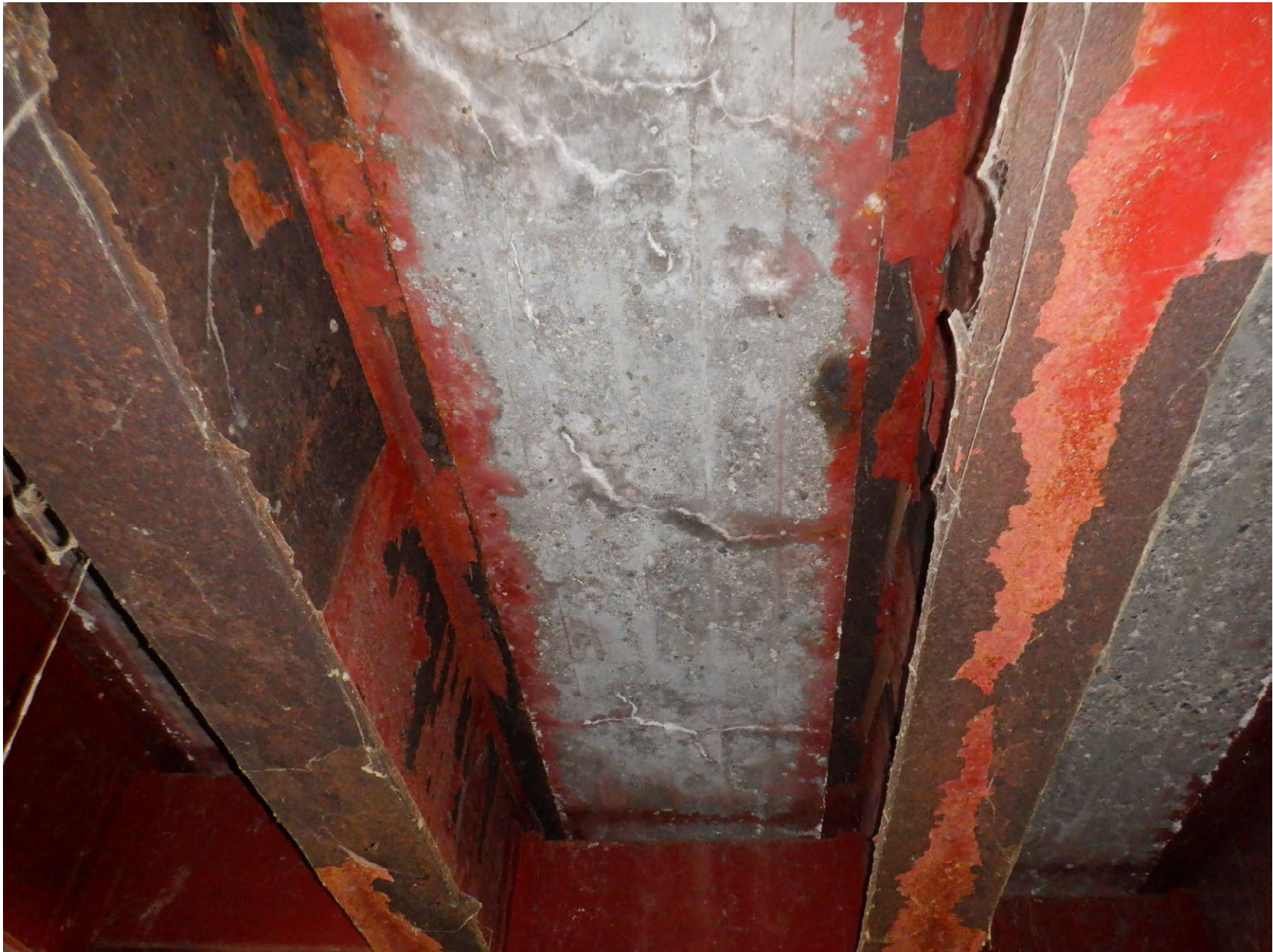
CRACKING WITH EFFLORESCENCE IN BOTTOM DECK SURFACE
