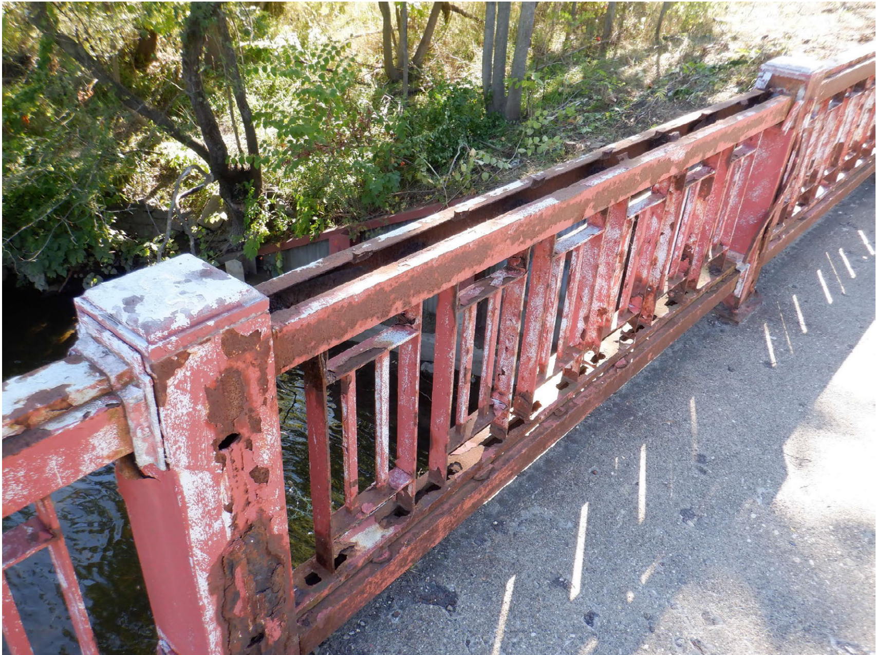
MISSING TOP RAIL COVER PLATE ON EAST SIDE
