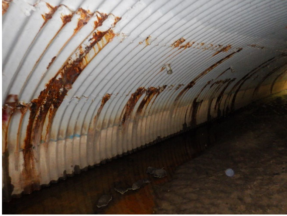
Corrosion inside culvert
