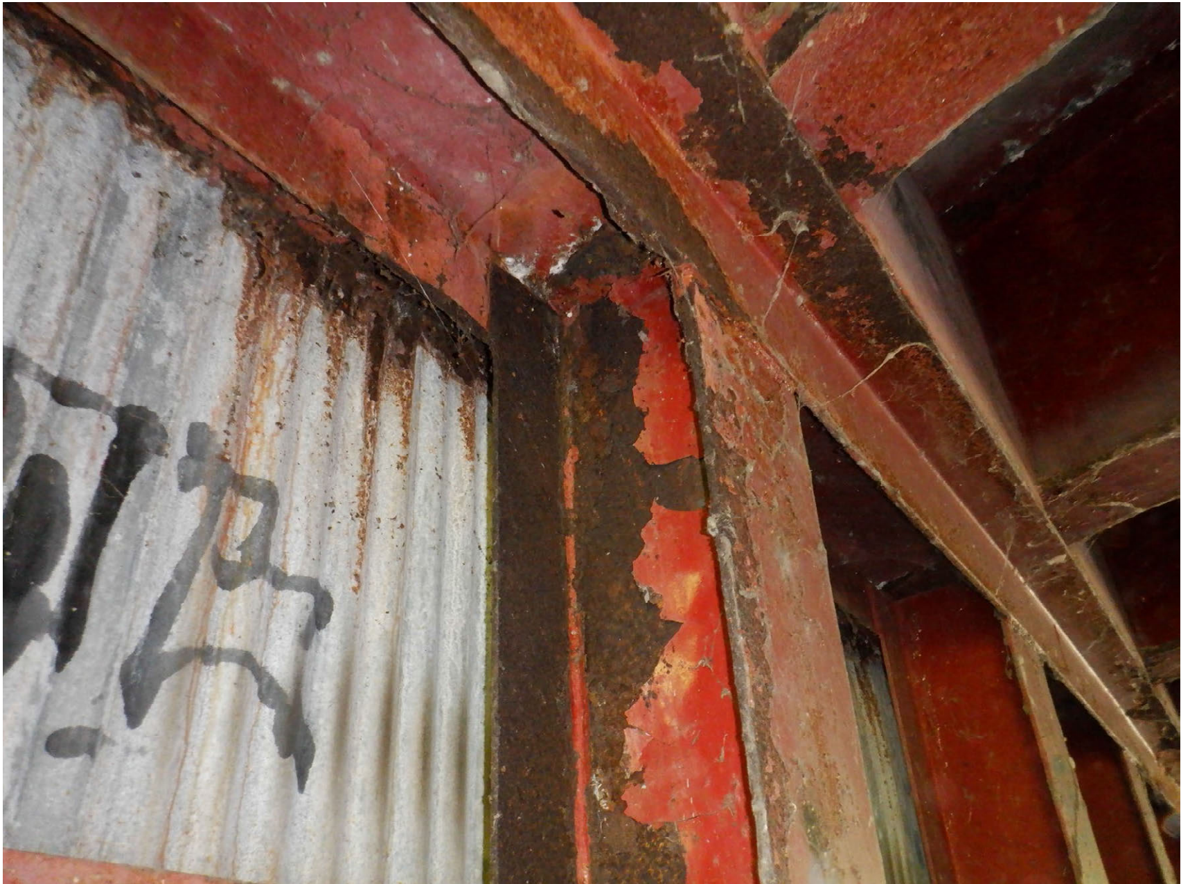
SECTION LOSS ON NORTH ABUTMENT PILE 4W
