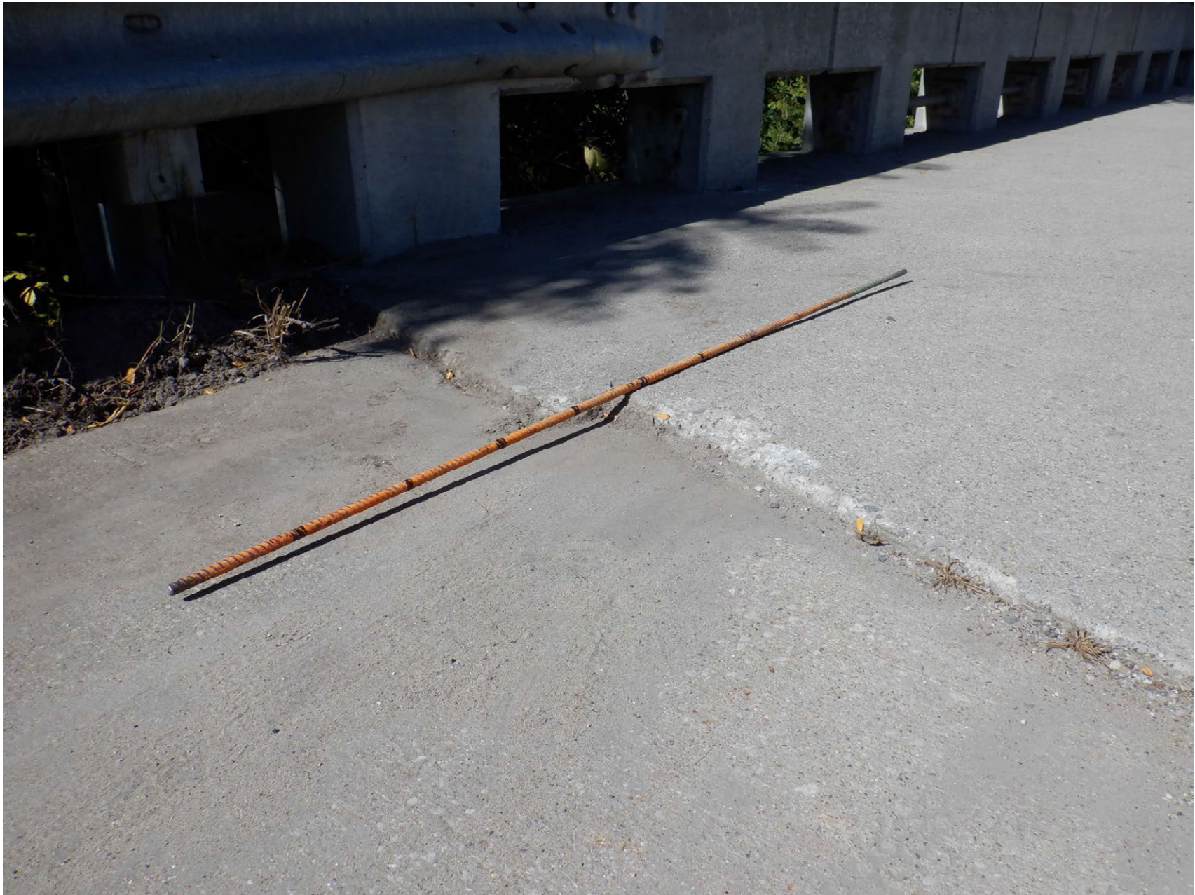
SIDEWALK SETTLED 1.25" IN SOUTHWEST QUAD
