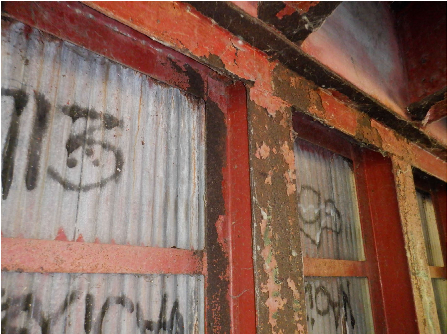
FLAKING PAINT AND RUST ON STEEL PILE AND HEADERS
