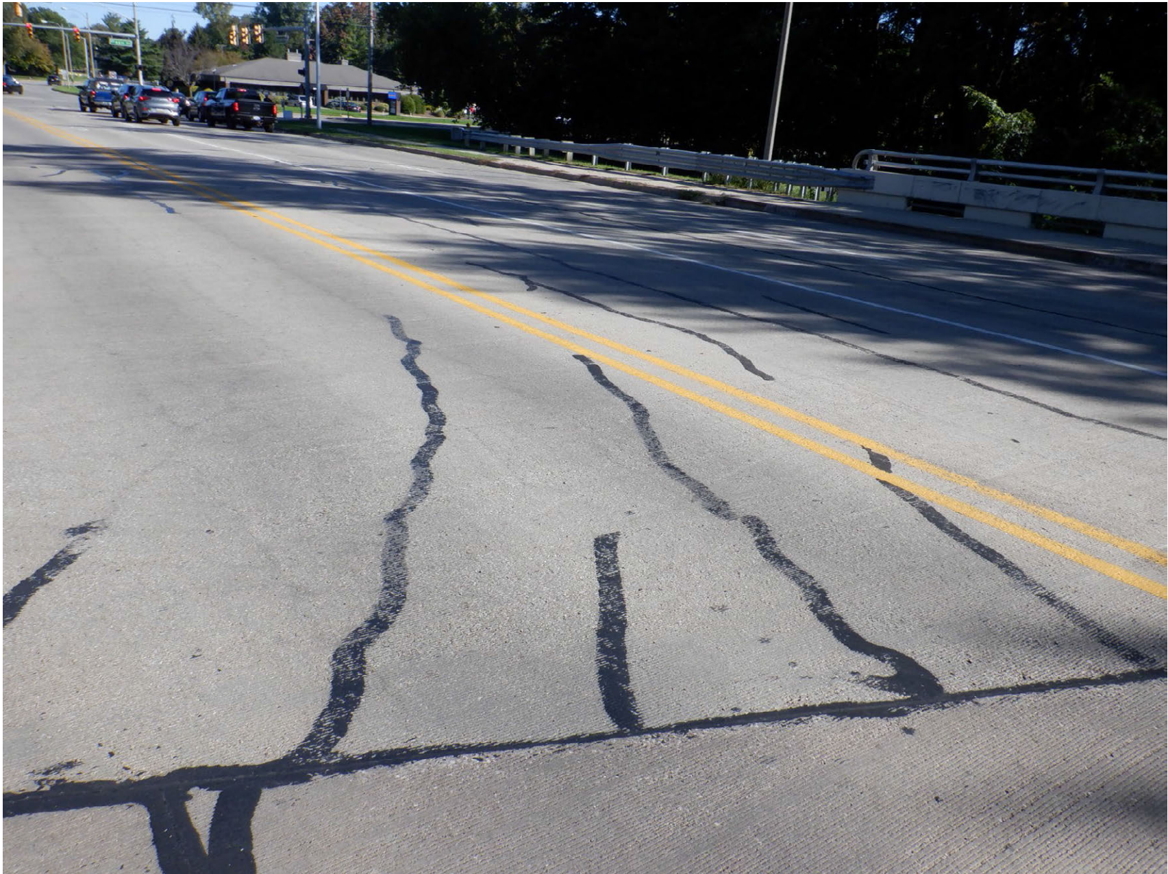
PREVIOUSLY SEALED CRACKS IN CONCRETE DECK SURFACE PERPENDICULAR TO SOUTH REFERENCE LINE
