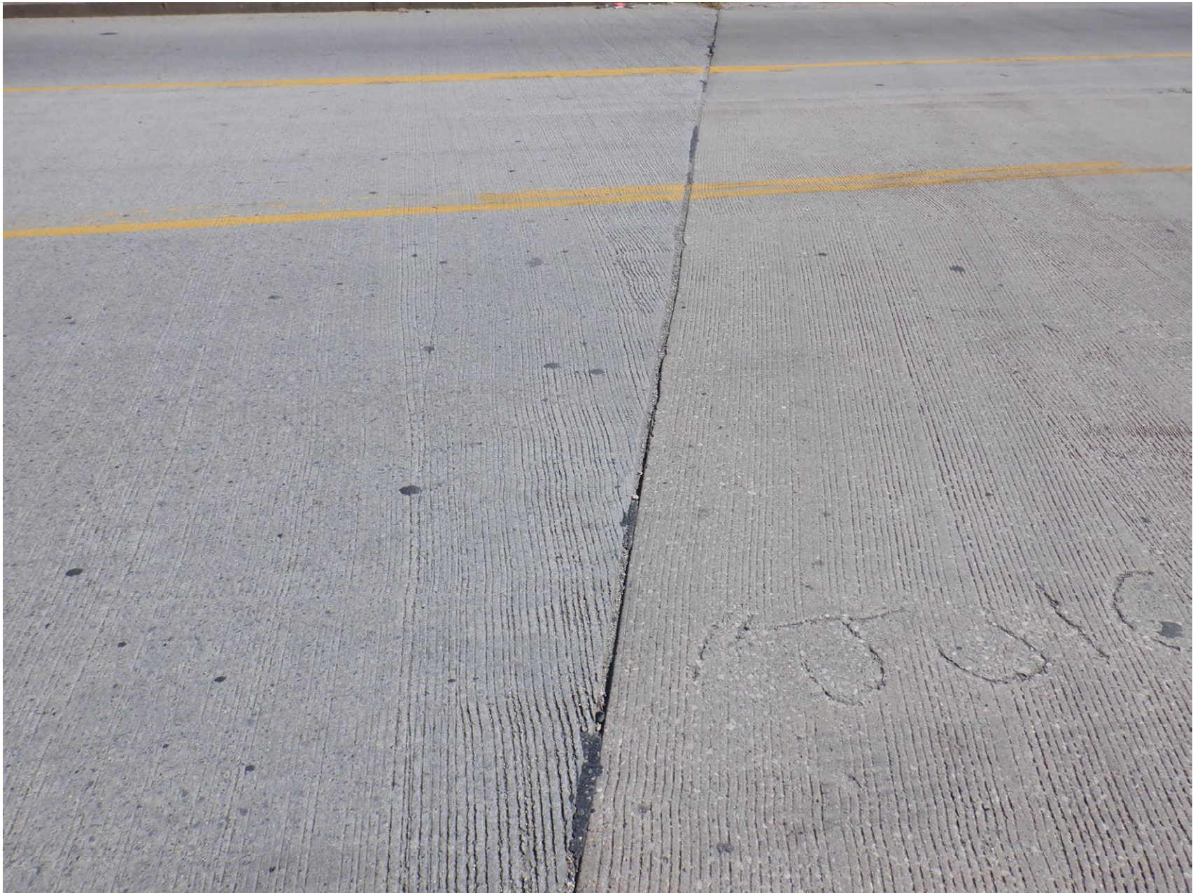
SEALANT MISSING ALONG SOUTH REFERENCE LINE JOINT
