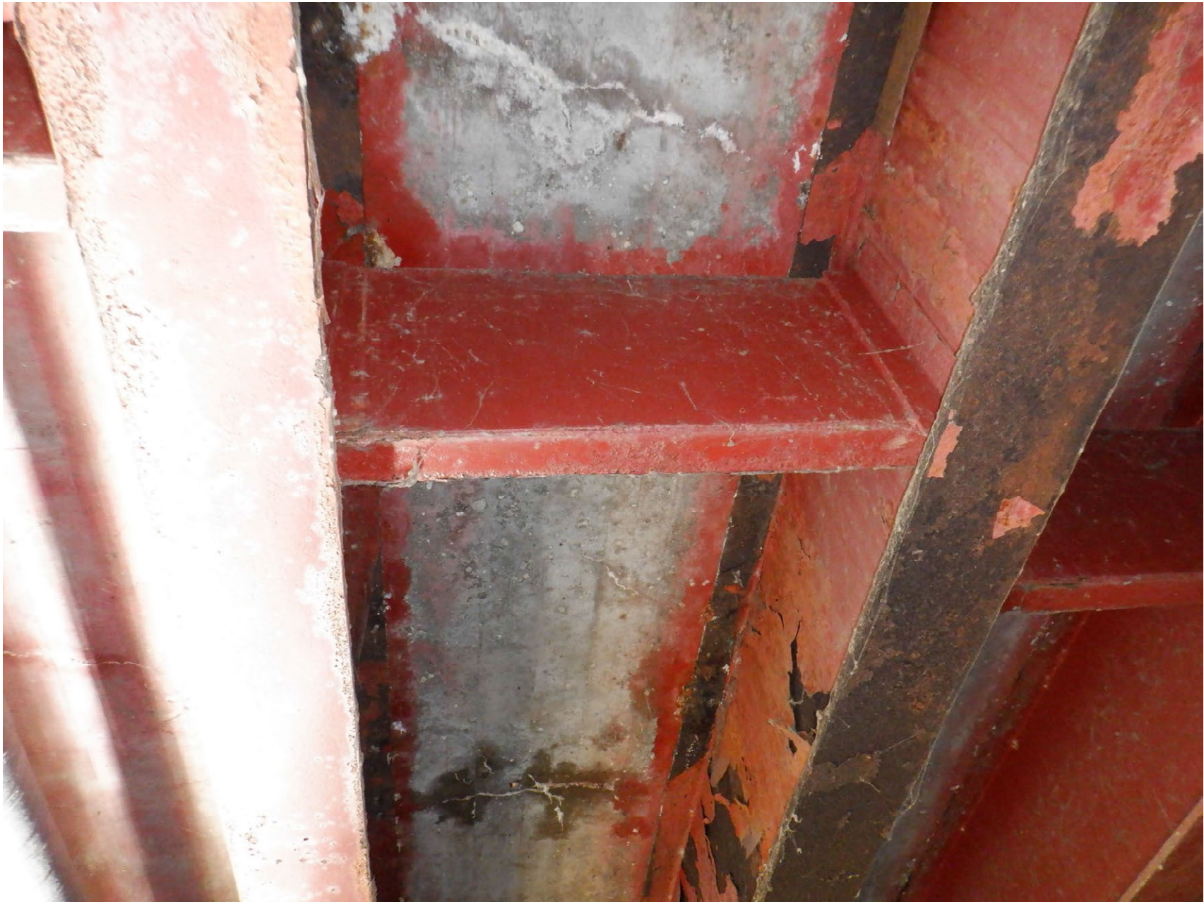
TRANSVERSE CRACKS WITH EFFLORESCENCE IN BOTTOM DECK SURFACE
