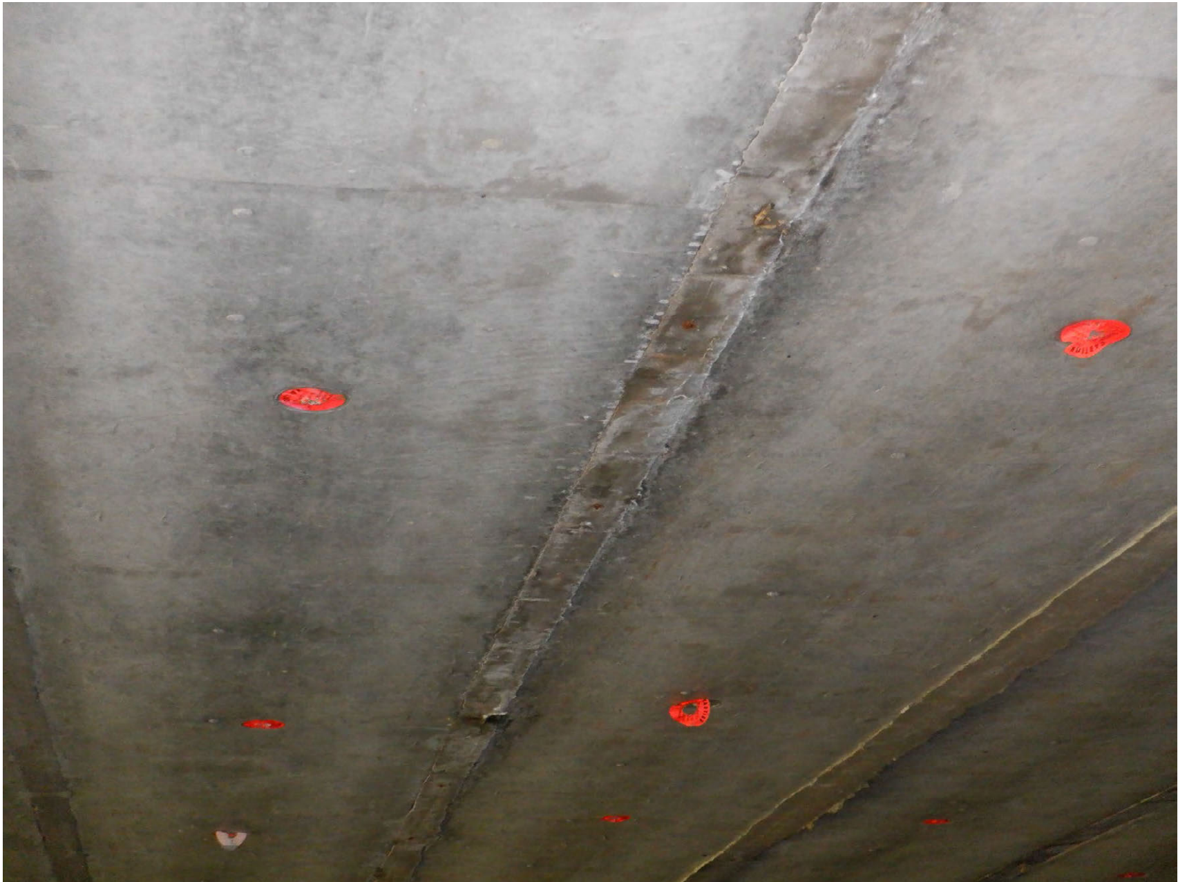
SPOT LEAKAGE AT BEAM JOINT
