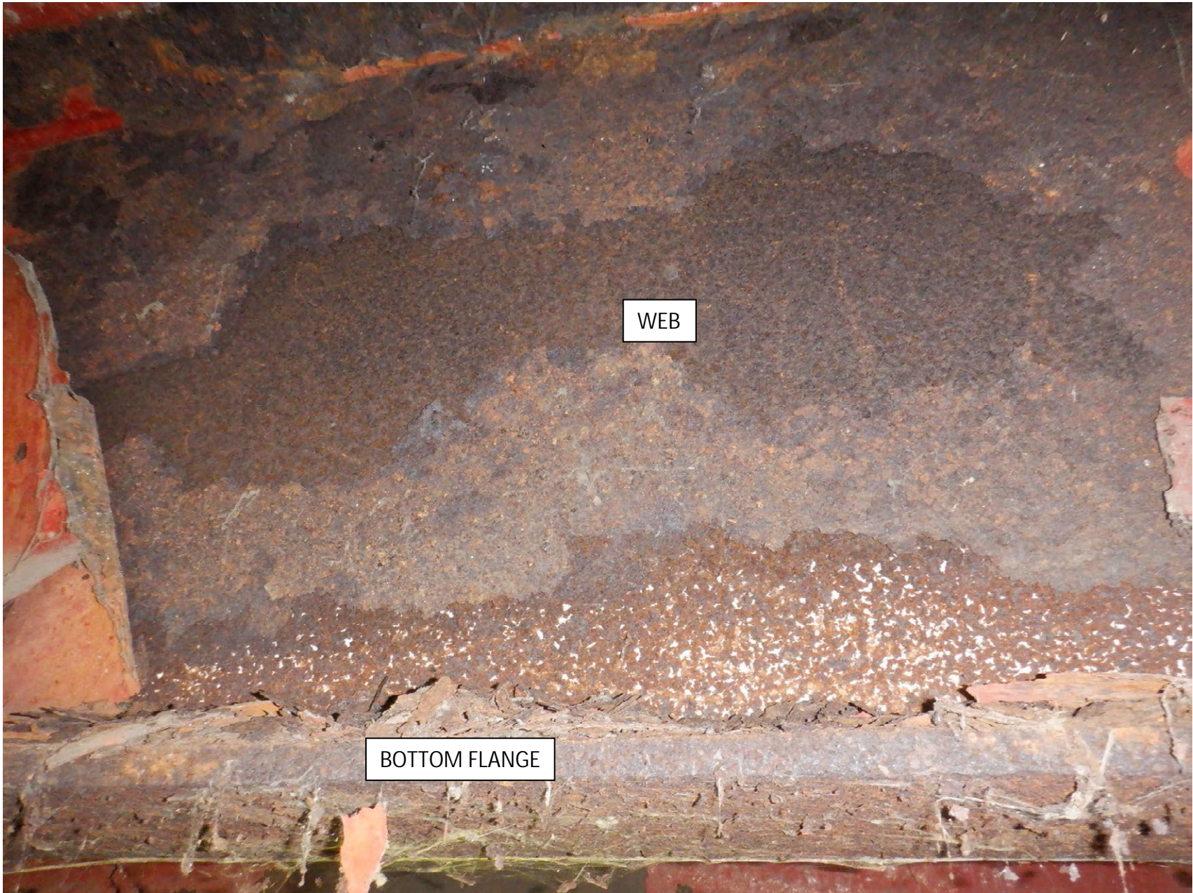
HEAVY SCALE ON CENTER BEAM NEAR NORTH ABUTMENT
