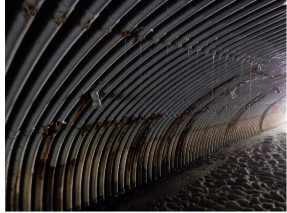
Leakage through culvert joints
