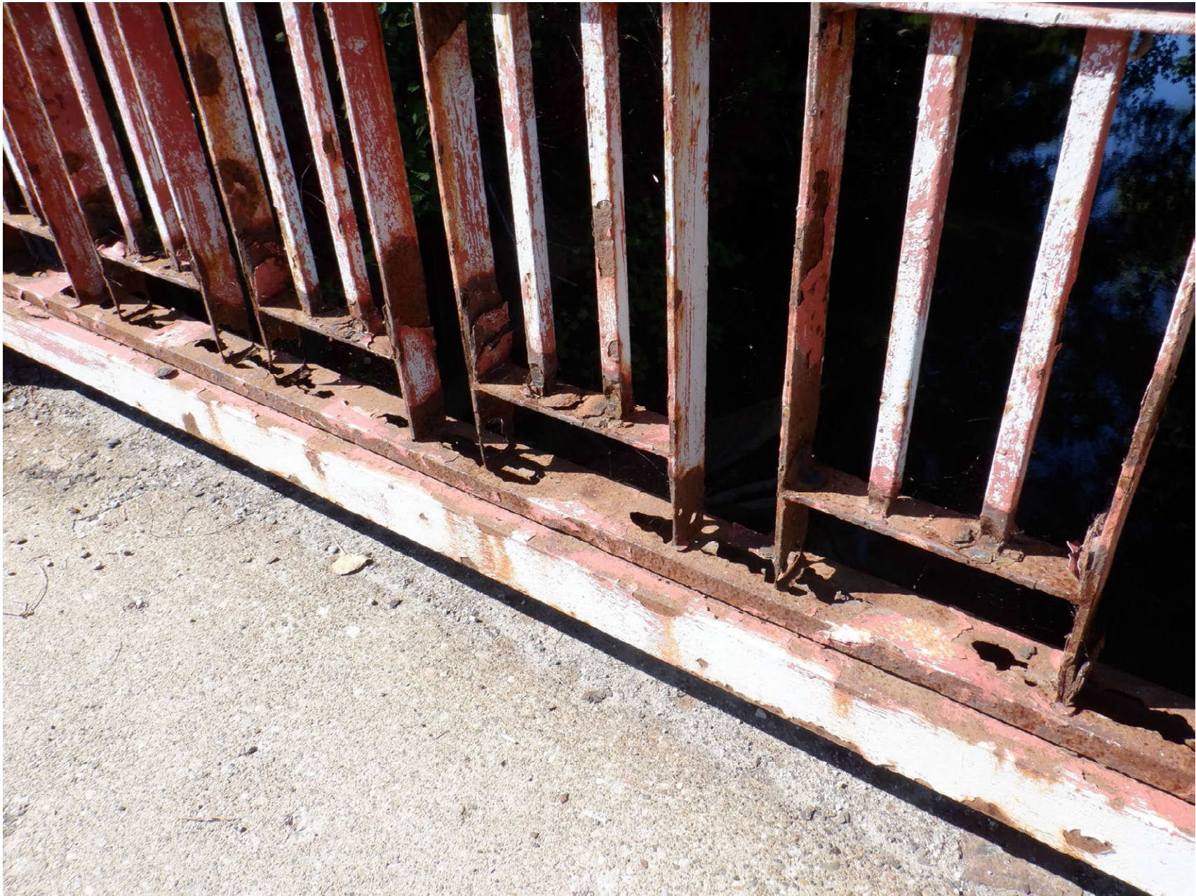
HOLES IN BOTTOM RAIL
