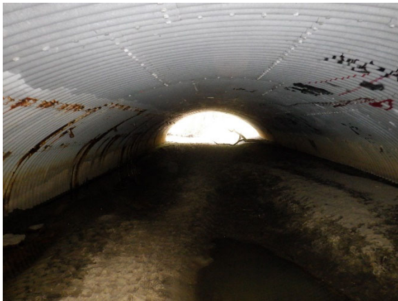
Sediment buildup in east barrel
