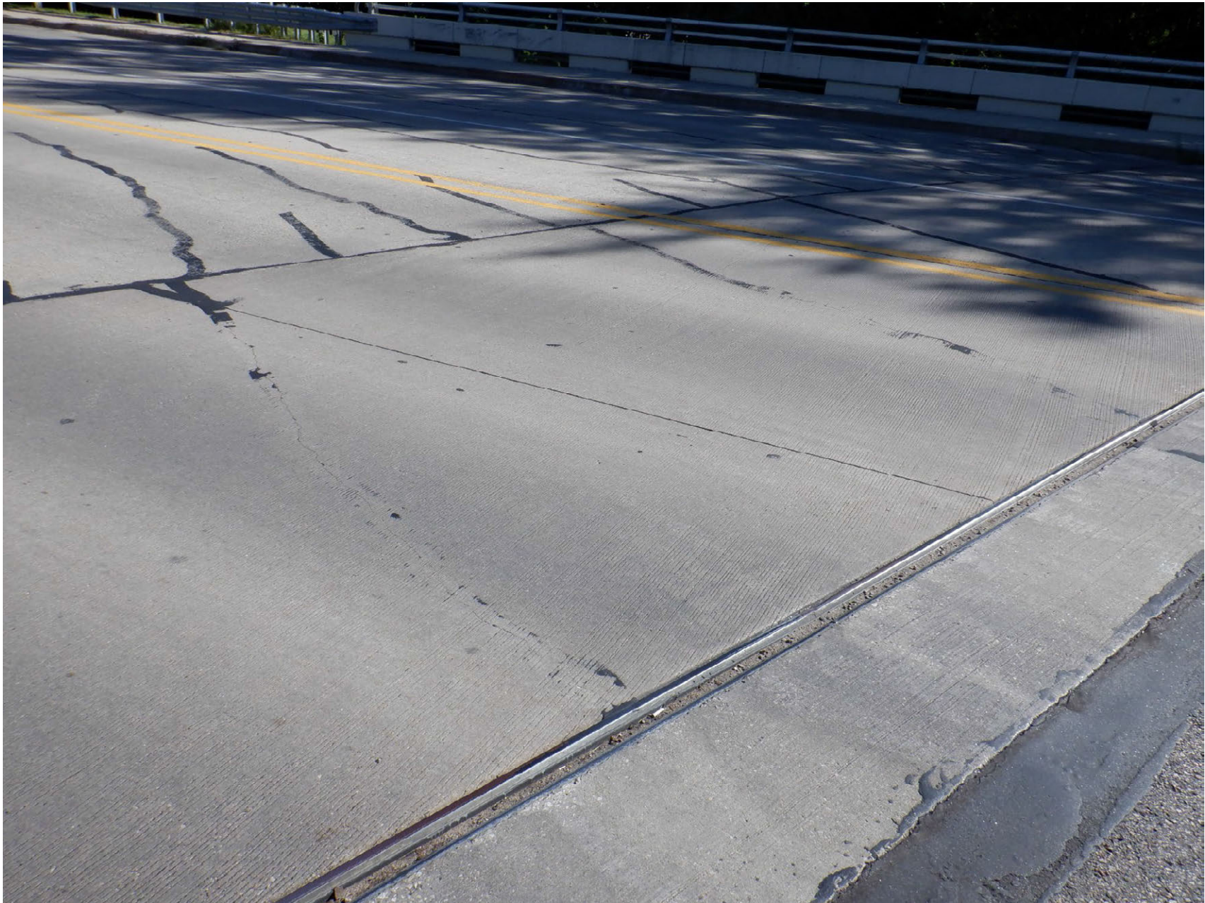
PREVIOUSLY SEALED CRACKS IN SOUTH APPROACH SLAB PERPENDICULAR TO JOINTS
