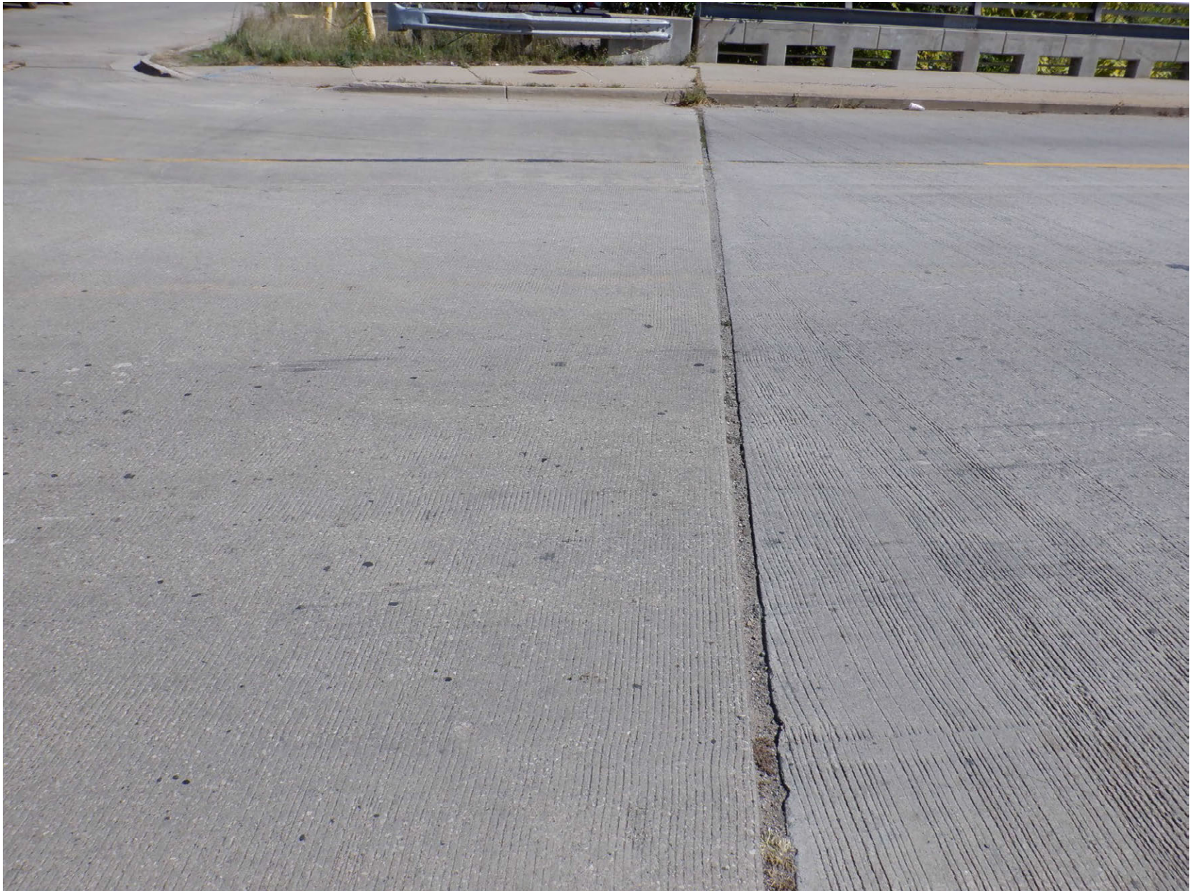
NORTH REFERENCE LINE JOINT FULL OF DIRT
