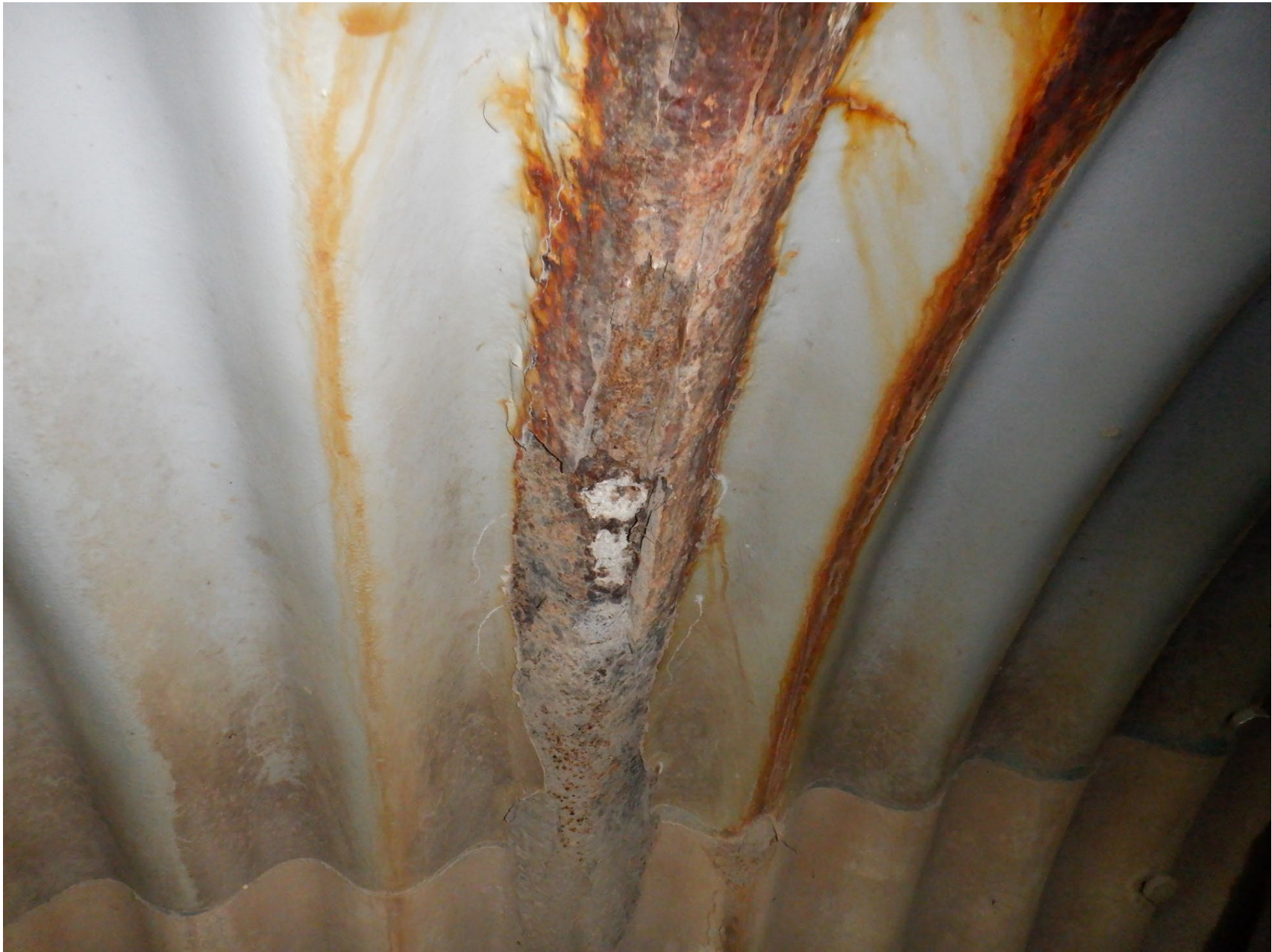
HOLE IN WEST WALL OF EAST BARREL WITH EXPOSED CONCRETE THRUST BLOCK, 40' FROM NORTH END
