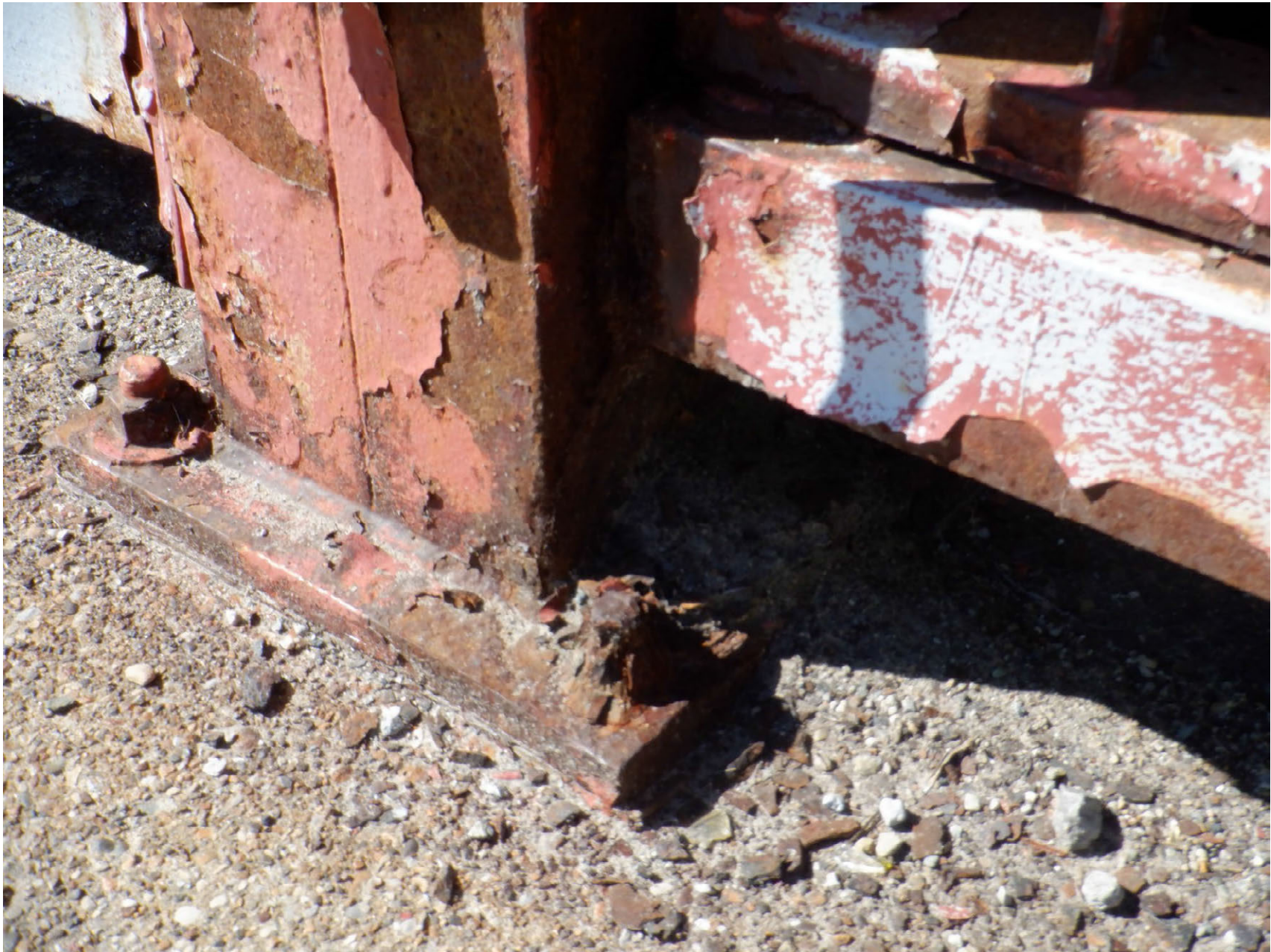
SEVERE SECTION LOSS TO NUT ON RAIL POST ANCHOR BOLT
