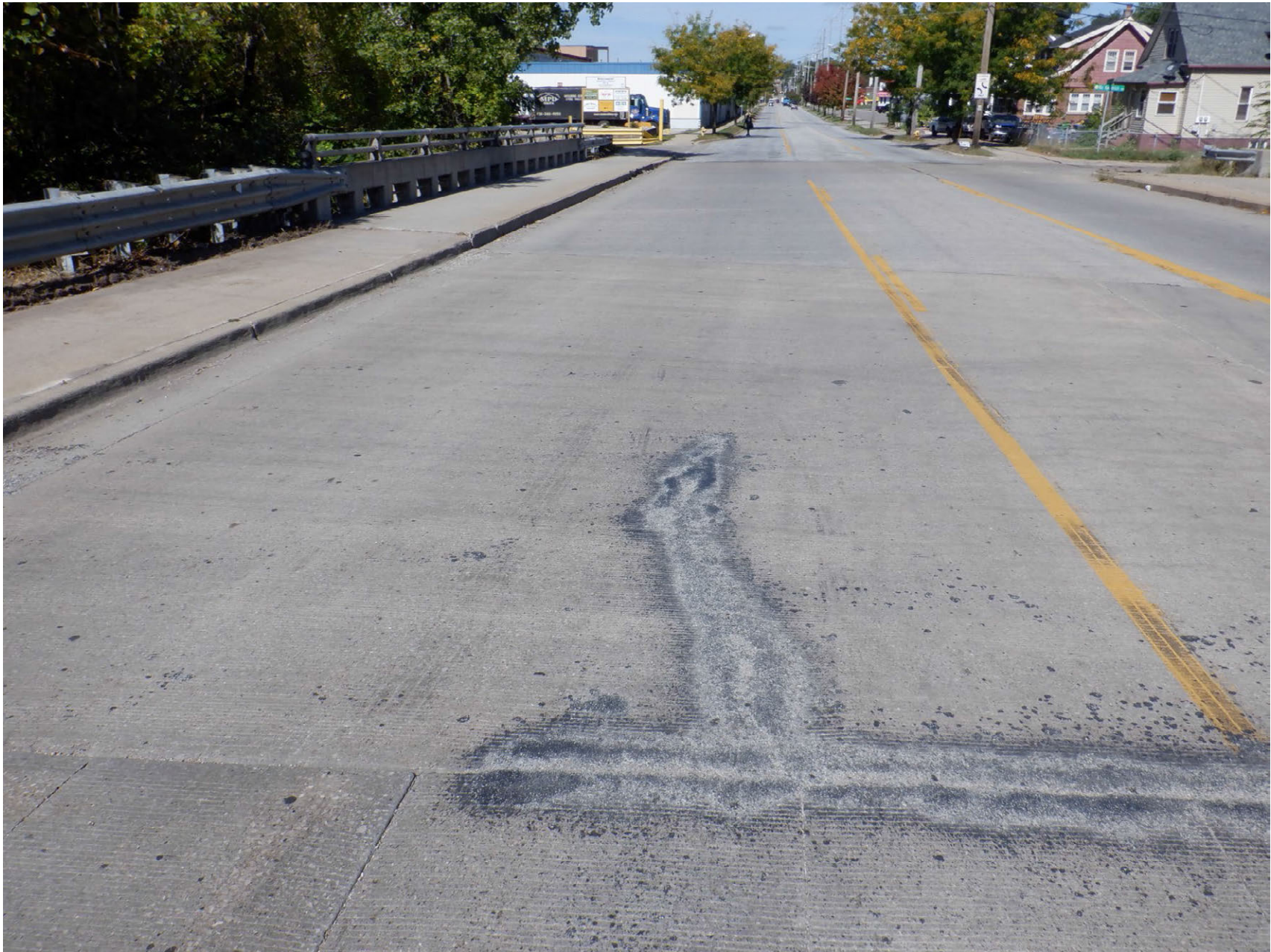
PATCHED CRACK AT SOUTH END OF SOUTH APPROACH SLAB IN SOUTHBOUND LANE
