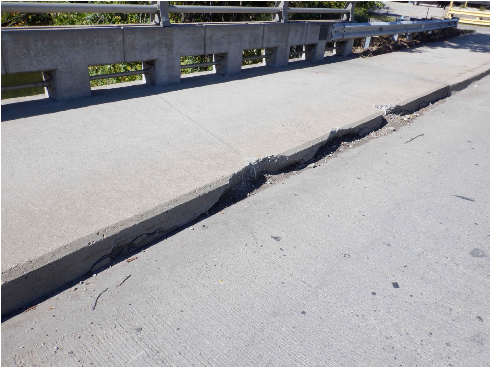
SPALLS WITH EXPOSED REBAR ALONG WEST SIDEWALK FACE
