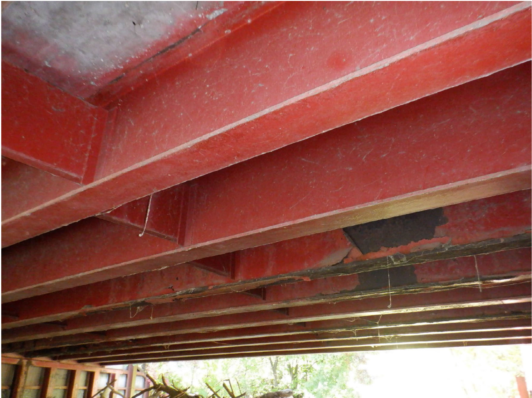
AREAS OF FLAKING PAINT AND CORROSION ON STEEL BEAMS
