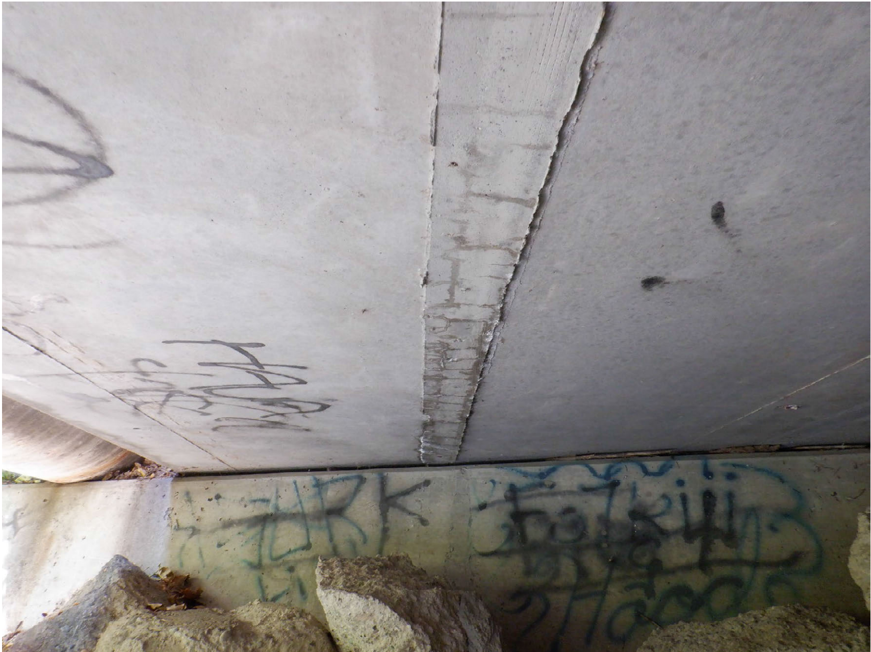
MINOR LEAKAGE AT NORTH END OF BEAM JOINT 1W
