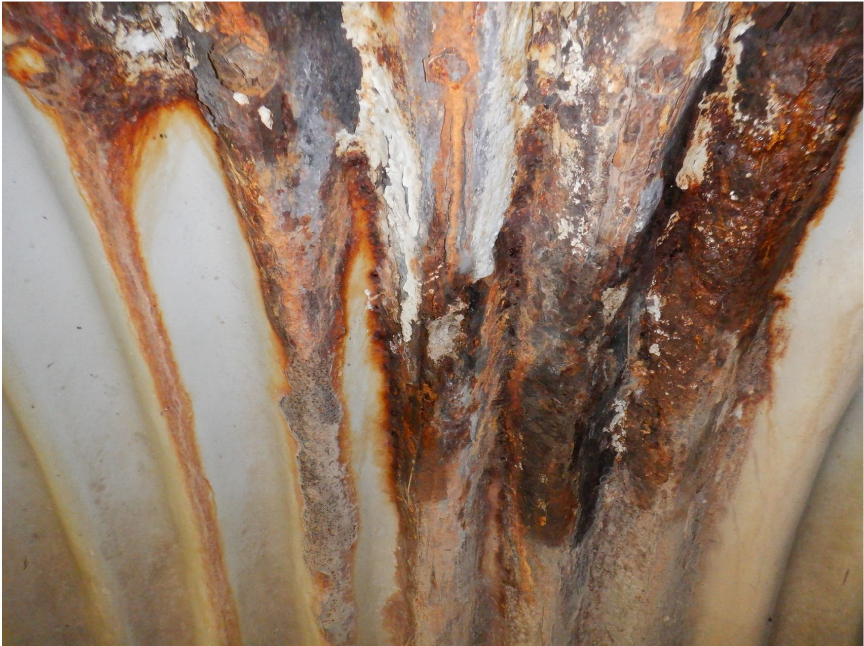
HOLE IN EAST WALL OF WEST BARREL
