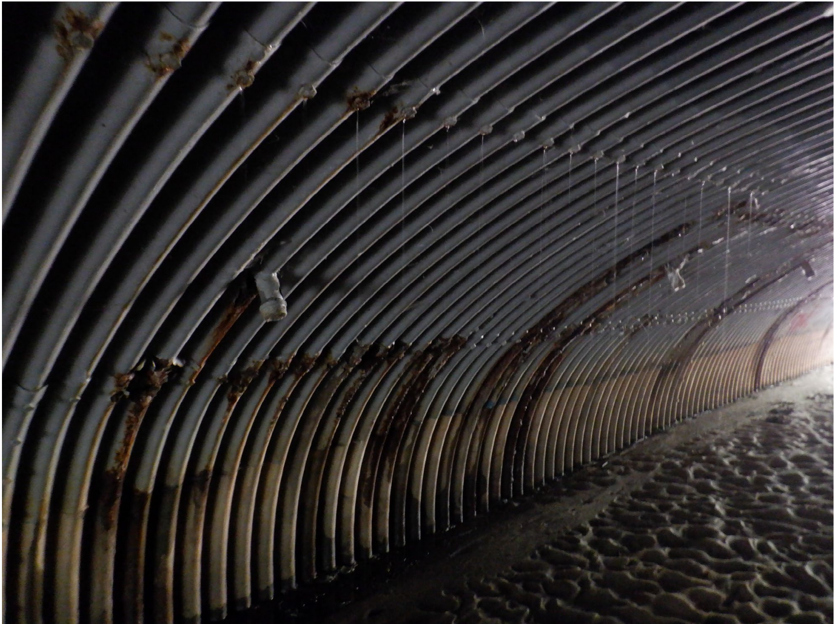
ACTIVE LEAKAGE THROUGH JOINT IN WEST WALL OF EAST BARREL UNDER MEDIAN
