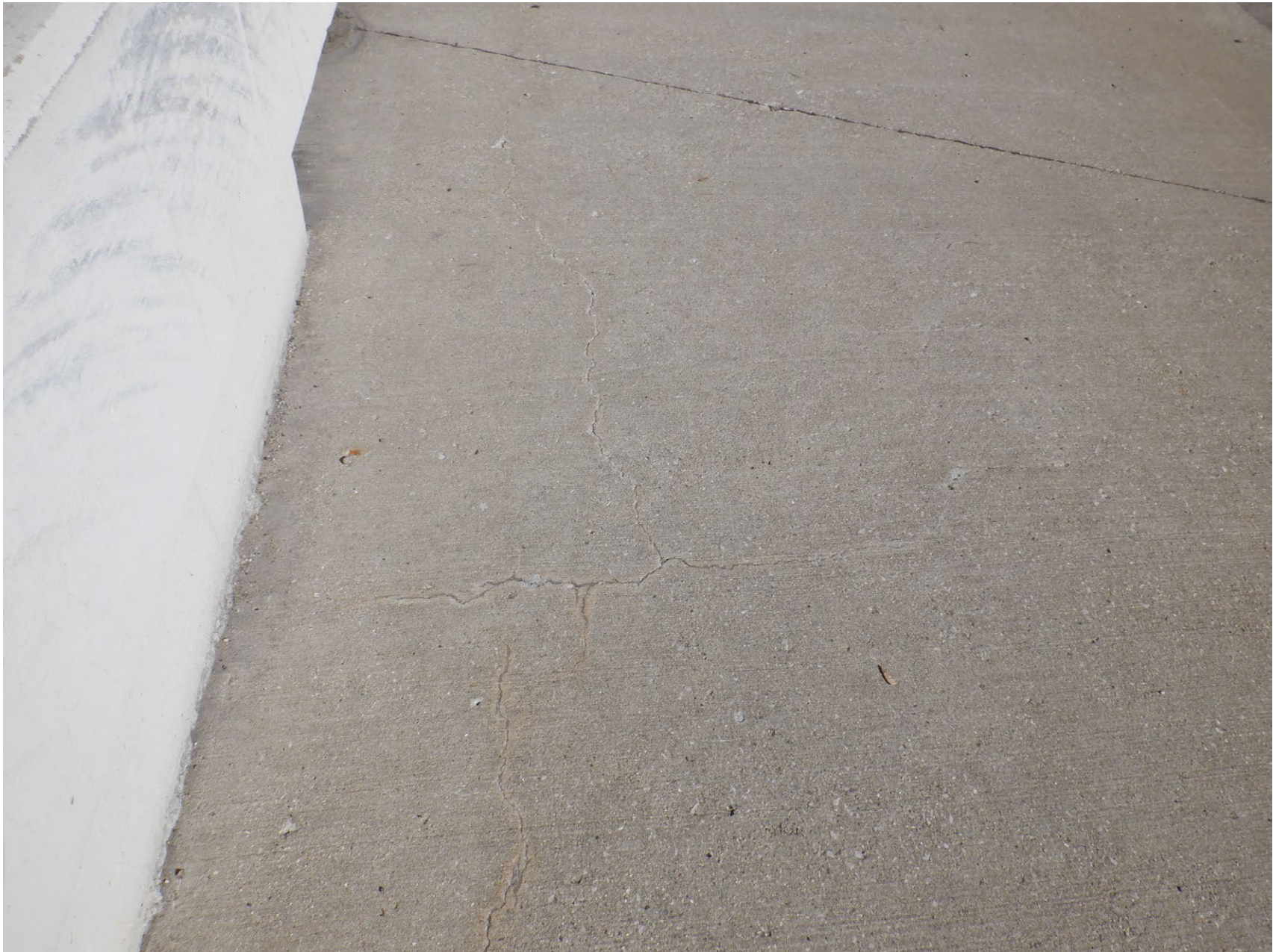
HAIRLINE LONGITUDINAL AND TRANSVERSE CRACKS IN SIDEWALK SURFACE
