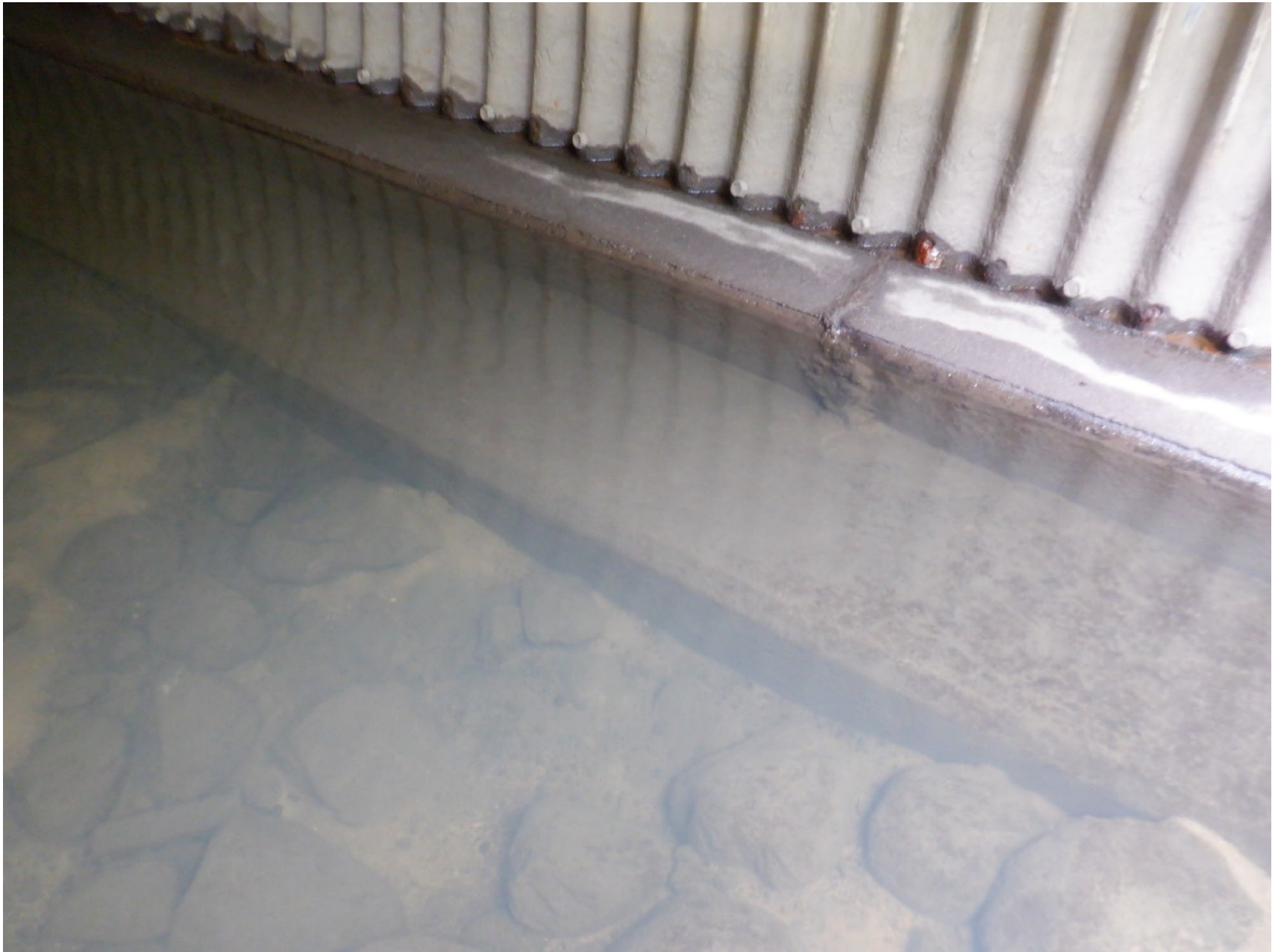
EXPOSED FOOTING ON WEST SIDE OF WEST BARREL AT NORTH END
