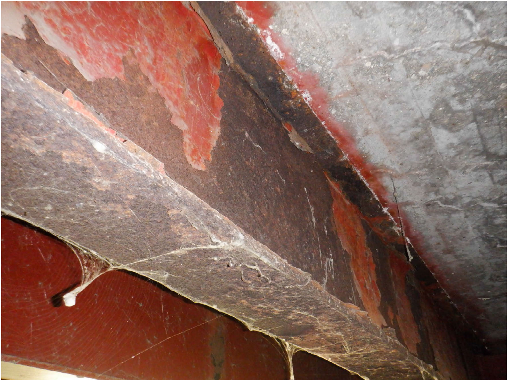
FLAKING PAINT AND CORROSION ON STEEL BEAM
