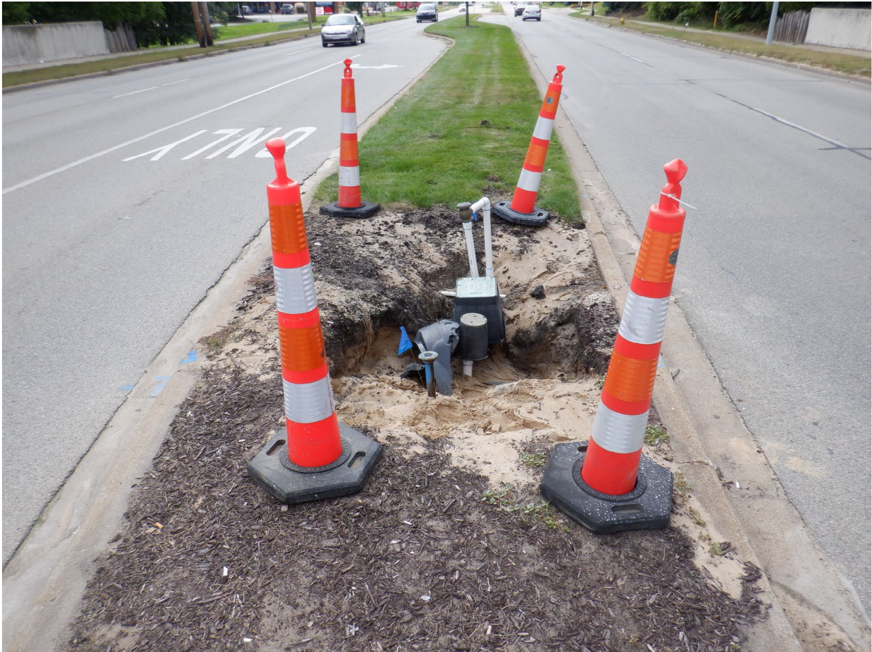
IRRIGATION SYSTEM REPAIRS IN MEDIAN
