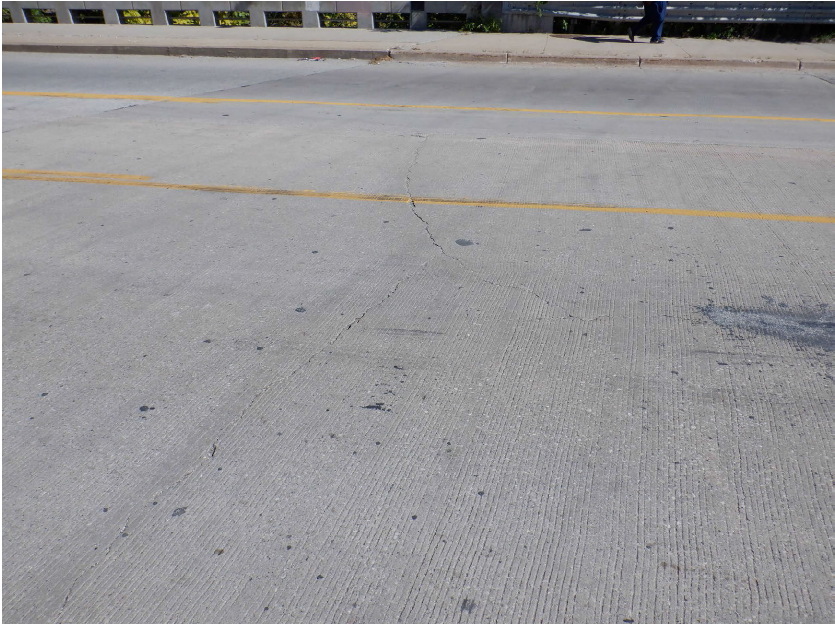
TRANSVERSE AND LONGITUDINAL CRACK IN SOUTH APPROACH SLAB
