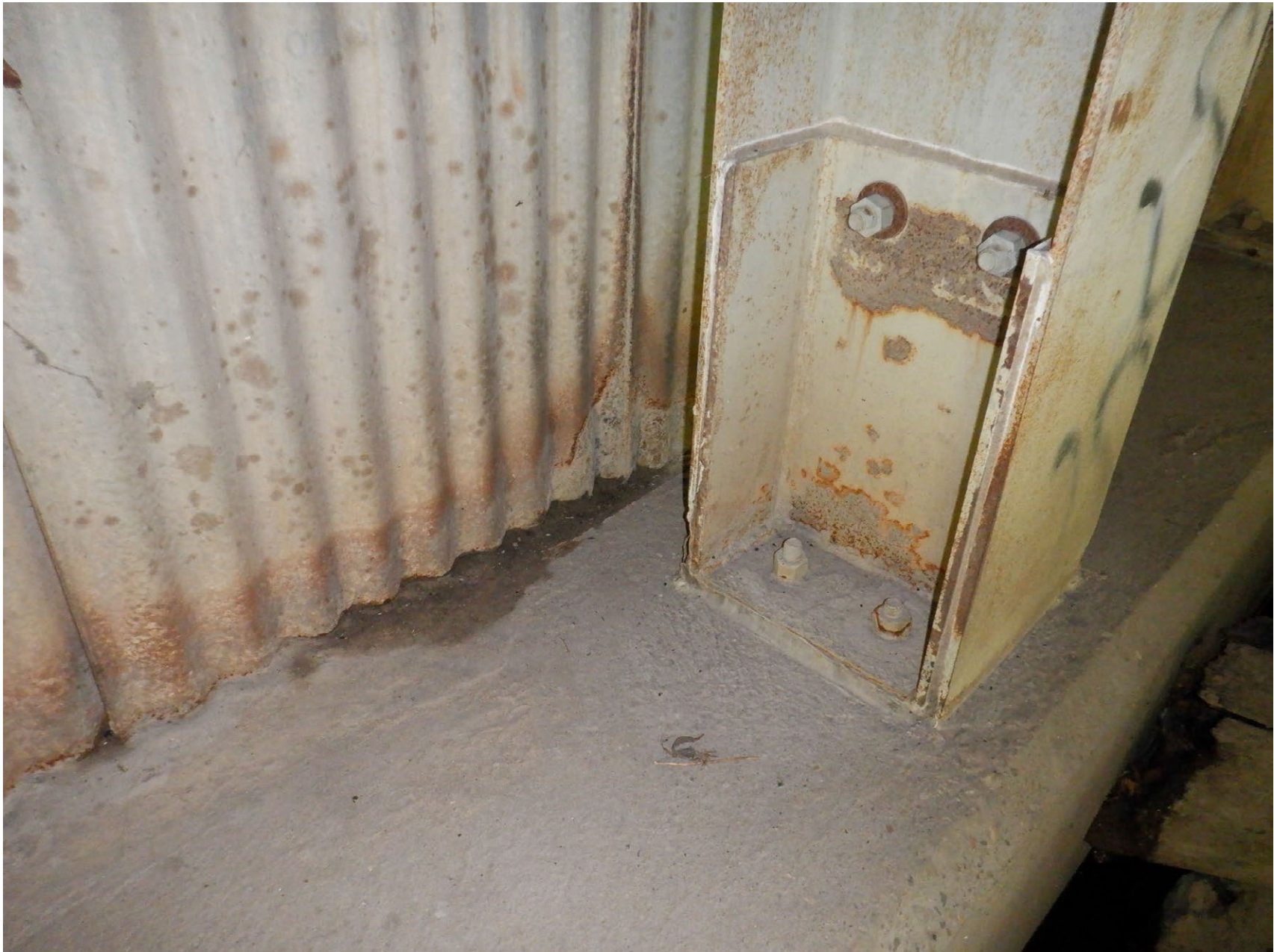
MINOR RUST ON REPAIR PLATE AT BOTTOM OF ABUTMENT PILE
