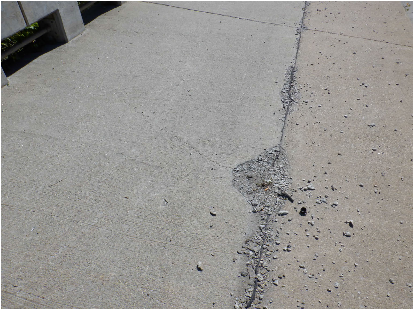
SPALLING IN EAST SIDEWALK SURFACE ALONG LONGITUDINAL JOINT
