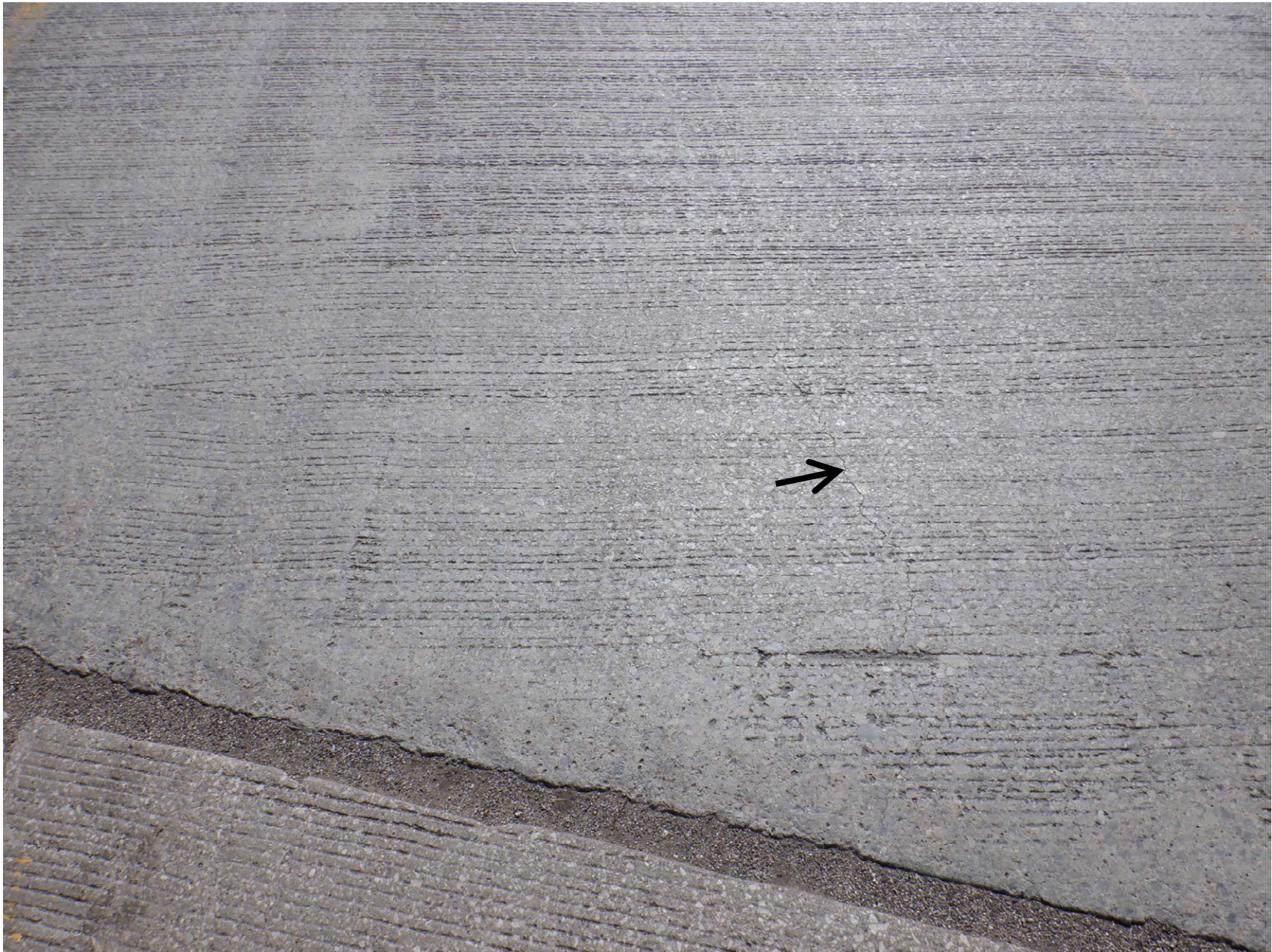
HAIRLINE CRACK IN CONCRETE DECK SURFACE AT NORTH END
