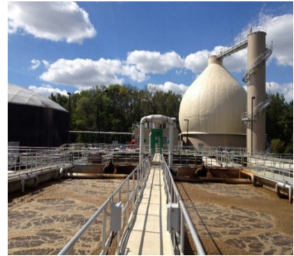
Egg-Shaped Anaerobic Digester
