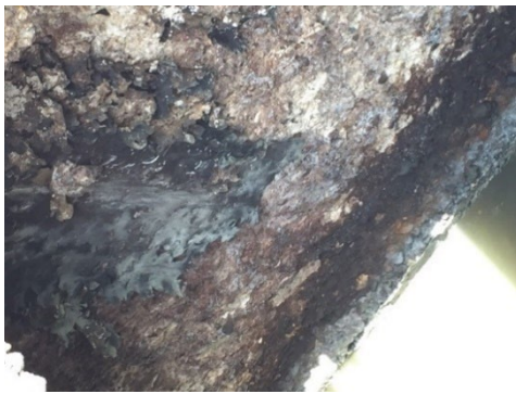
Failed Concrete on Channel
