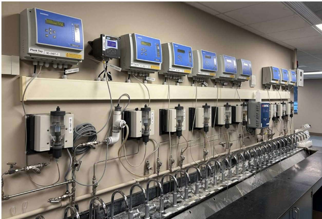
Current Online Chlorine Analyzers at the Donald K. Shine Drinking Water Plant.
