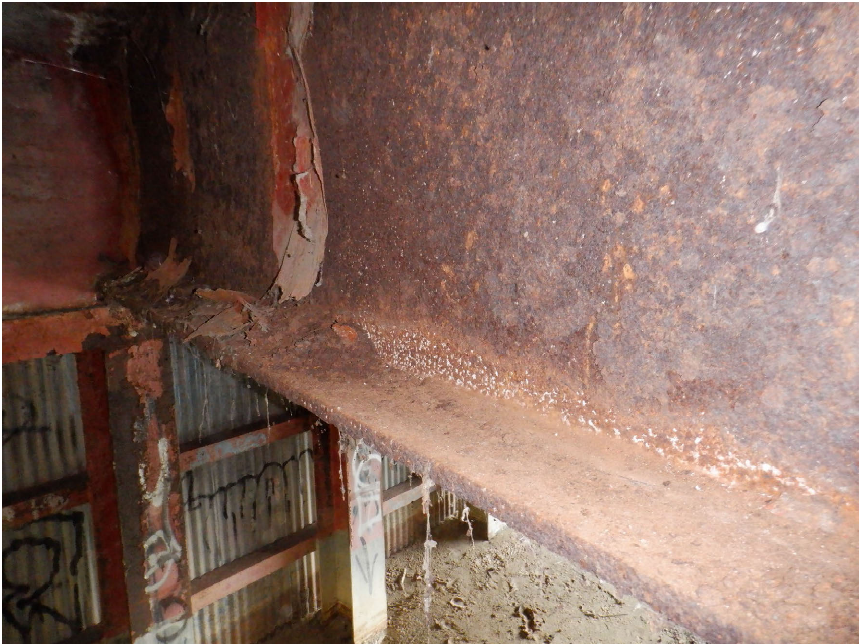
SECTION LOSS ON BOTTOM FLANGE AND WEB OF BEAM 7E AT NORTH END
