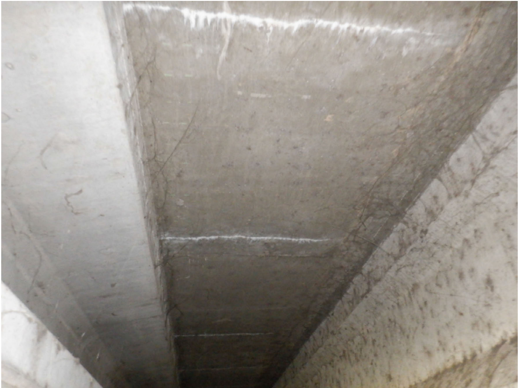
HAIRLINE TRANSVERSE CRACKS IN BOTTOM OF DECK, BAY 3N
