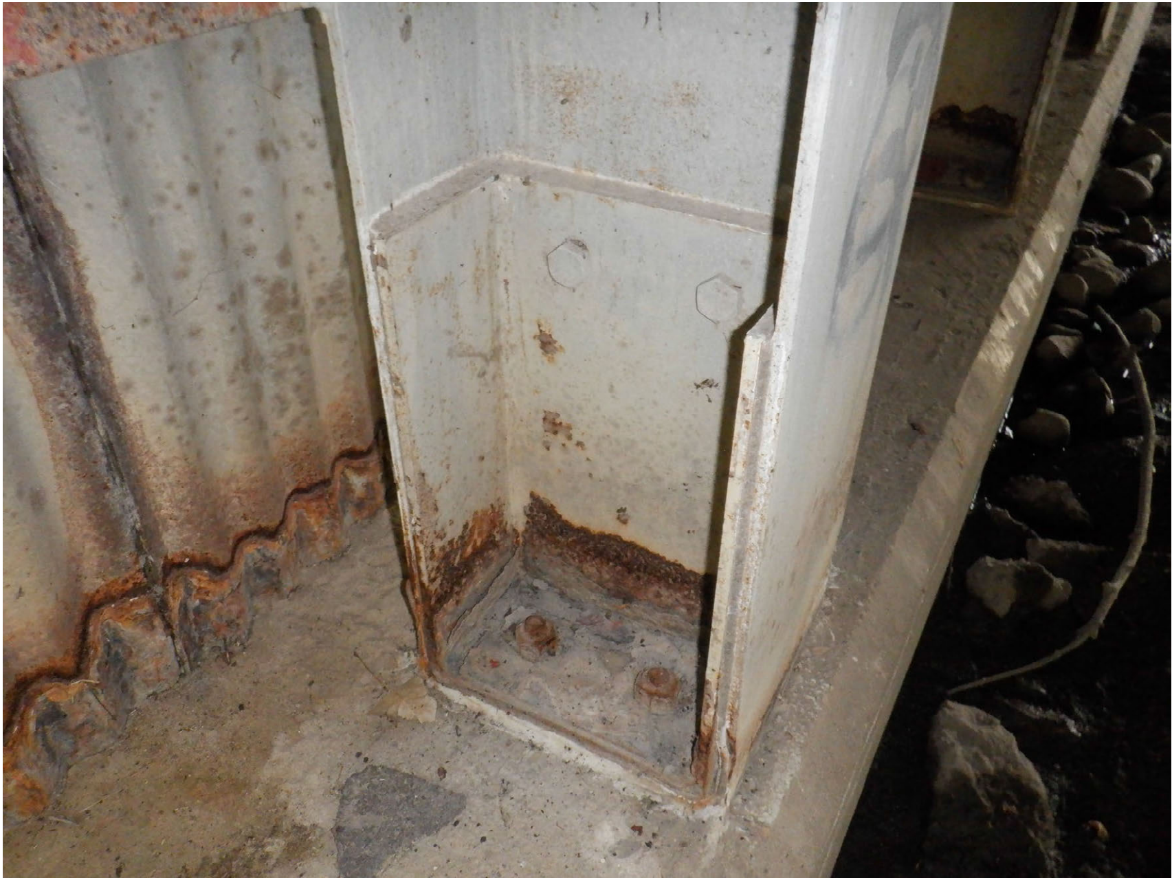
CORROSION ON STEEL PILE REPAIR
