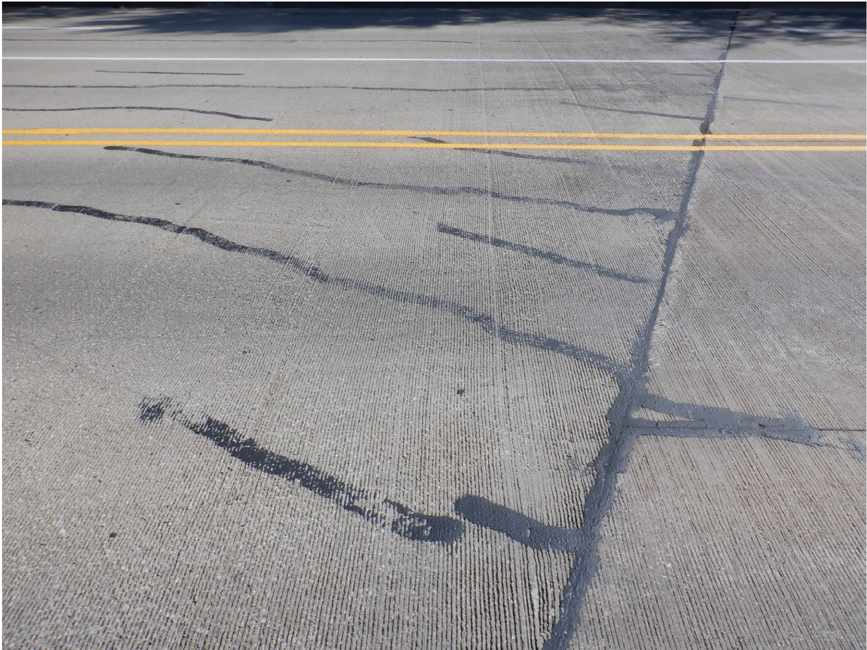
HAIRLINE CRACKS IN CONCRETE DECK PERPENDICULAR TO JOINT AND ALONG BEAM LINES, SOME PREVIOUSLY SEALED
