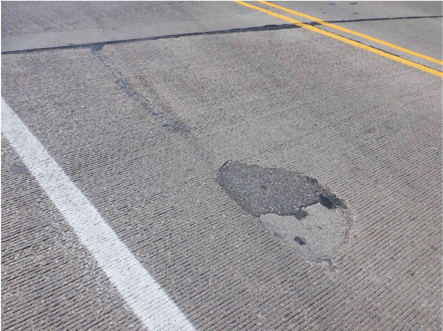
LONGITUDINAL CRACK AND PATCHED SPALL IN NORTH APPROACH SLAB
