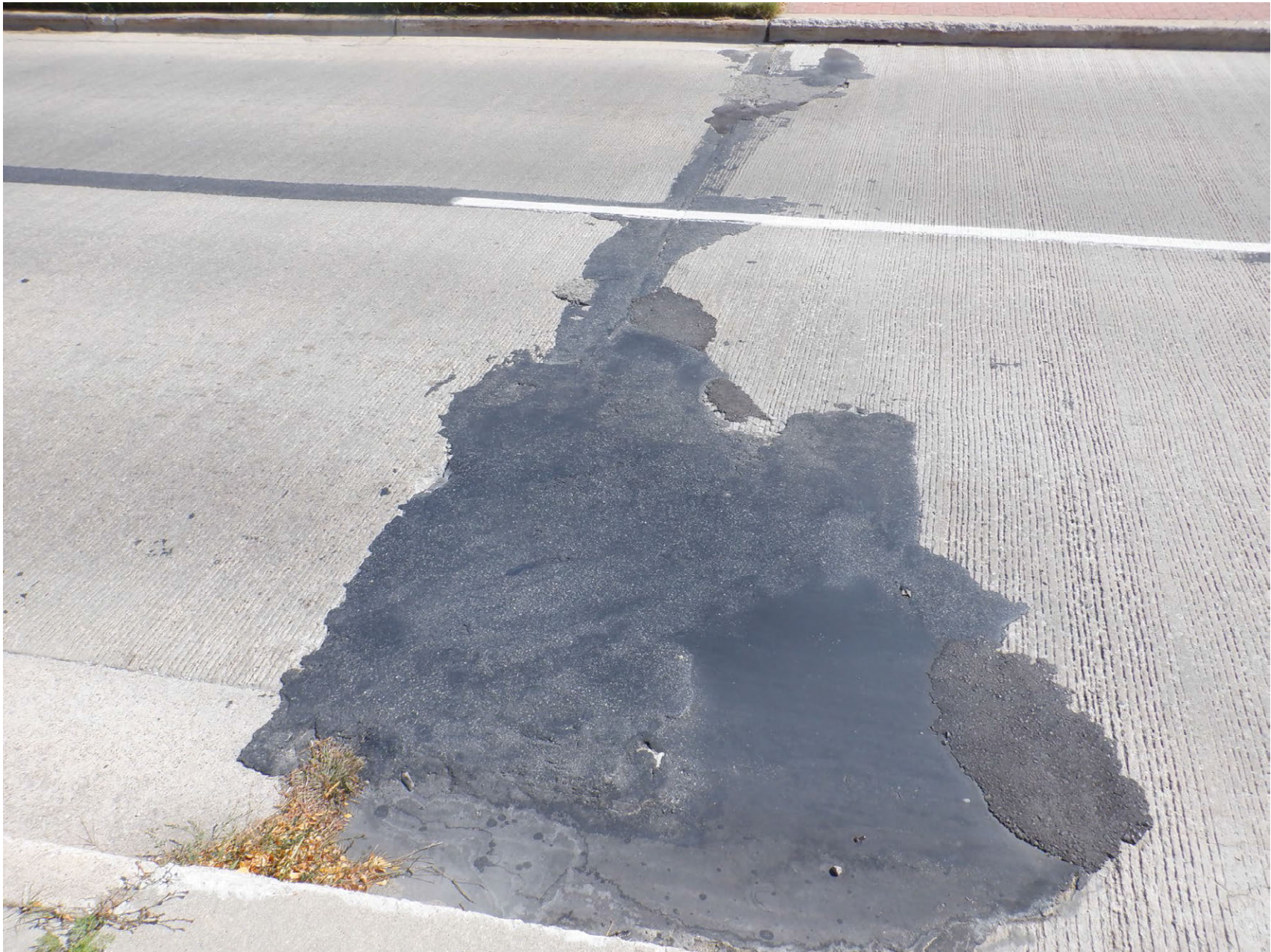
PATCHED SPALLS AT NORTH END OF DECK IN SOUTHBOUND LANES
