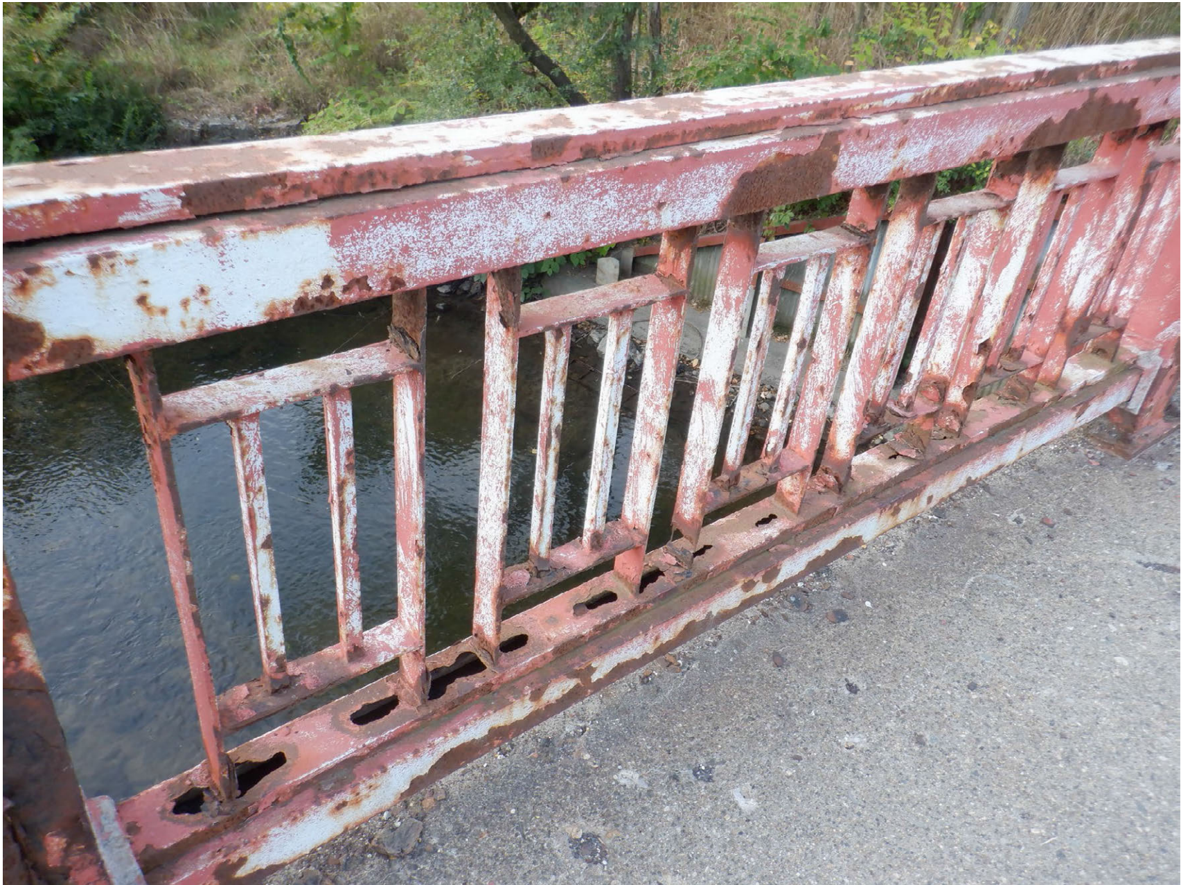
HEAVY CORROSION ON RAIL, HOLES ALONG BOTTOM RAIL
