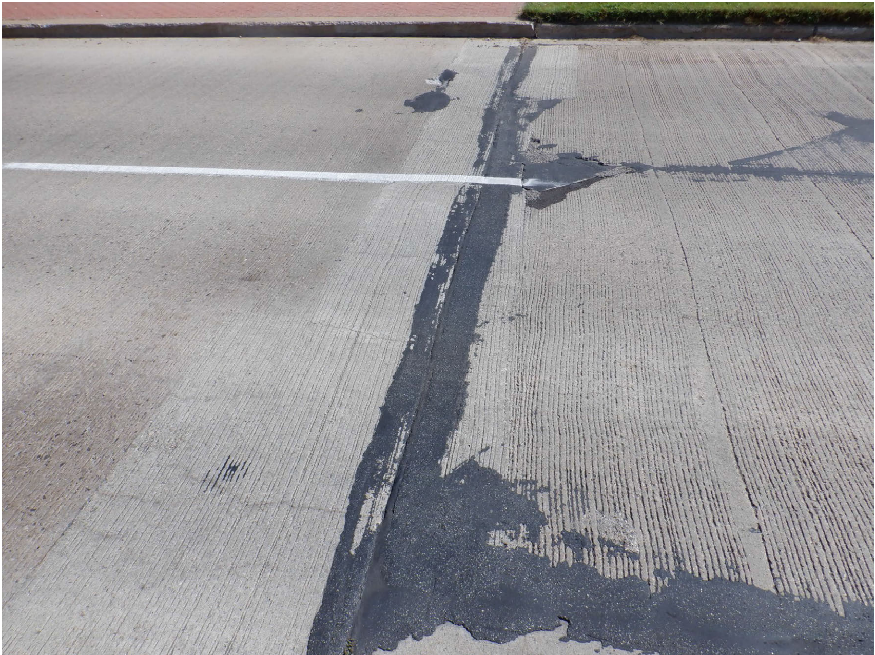
RUBBER SEAL AND PATCHES AT SOUTH REFERENCE LINE, PATCHED DECK SPALL INSIDE SOUTHBOUND LANE
