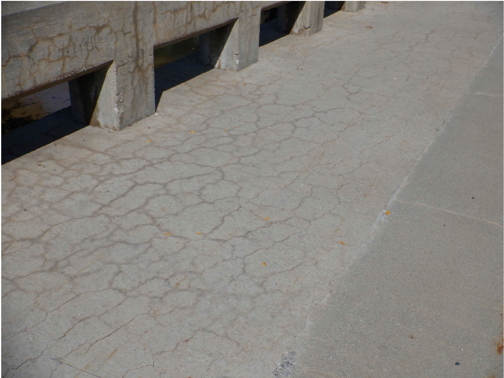
SHRINKAGE OR ASR CRACKING IN CONCRETE SIDEWALK
