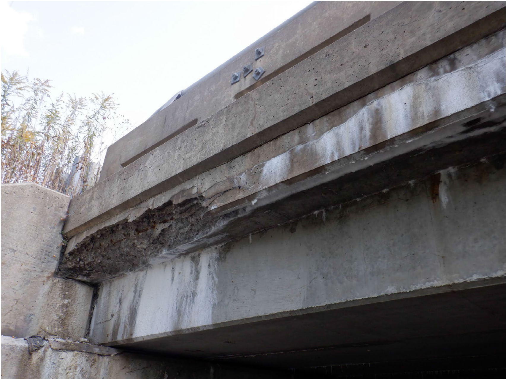
SPALL WITH EXPOSED REBAR AND HORIZONTAL CRACK WITH EFFLORESCENCE AT NORTH END OF WEST DECK FASCIA
