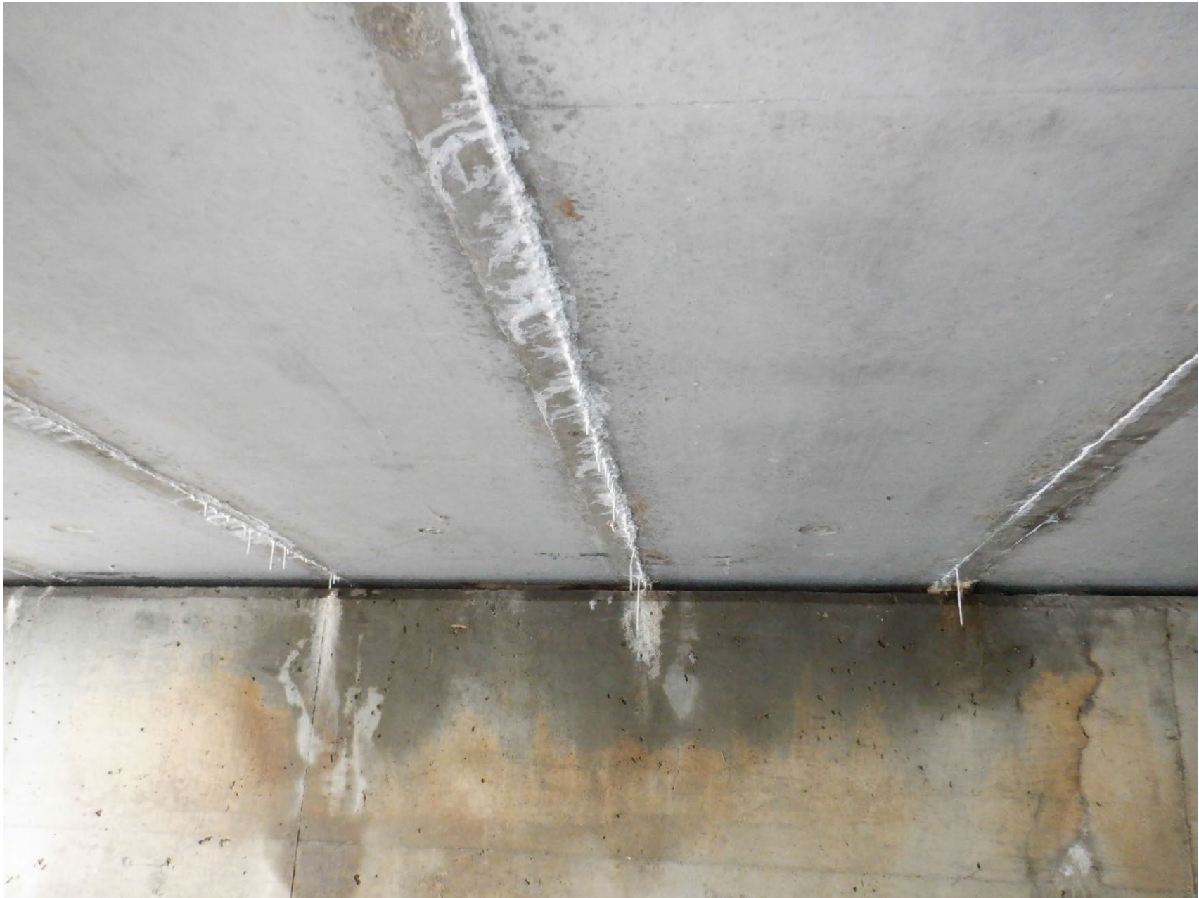
EFFLORESCENCE THROUGH BEAM JOINTS AT ABUTMENT
