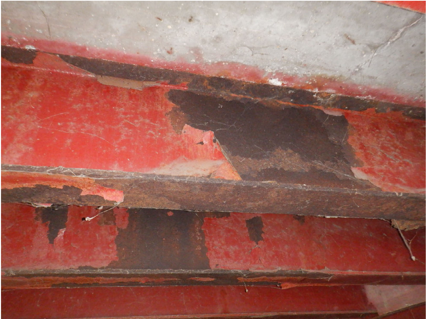
FLAKING PAINT AND CORROSION ON BEAMS NEAR CENTERLINE
