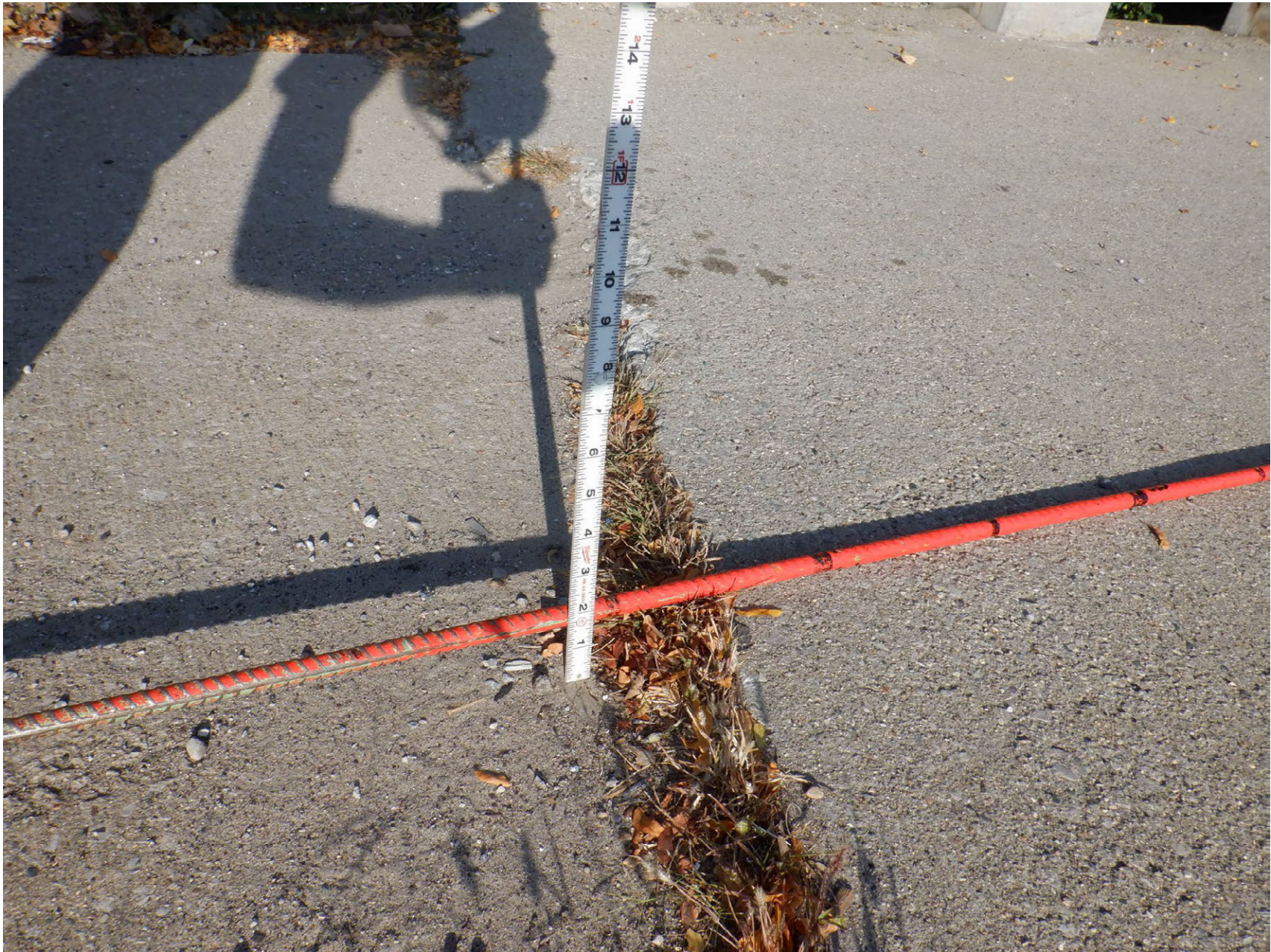
SOUTHWEST APPROACH SIDEWALK SETTLED 1.5" AT REFERENCE LINE
