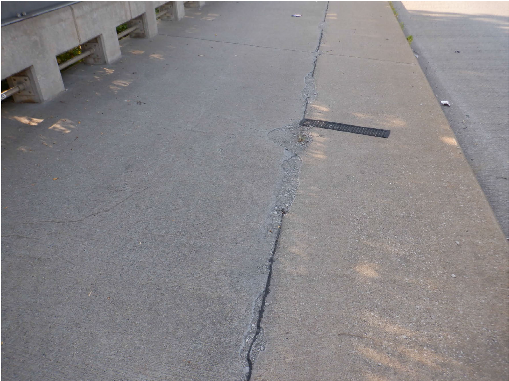
SHALLOW SPALLING ALONG LONGITUDINAL JOINT IN EAST SIDEWALK
