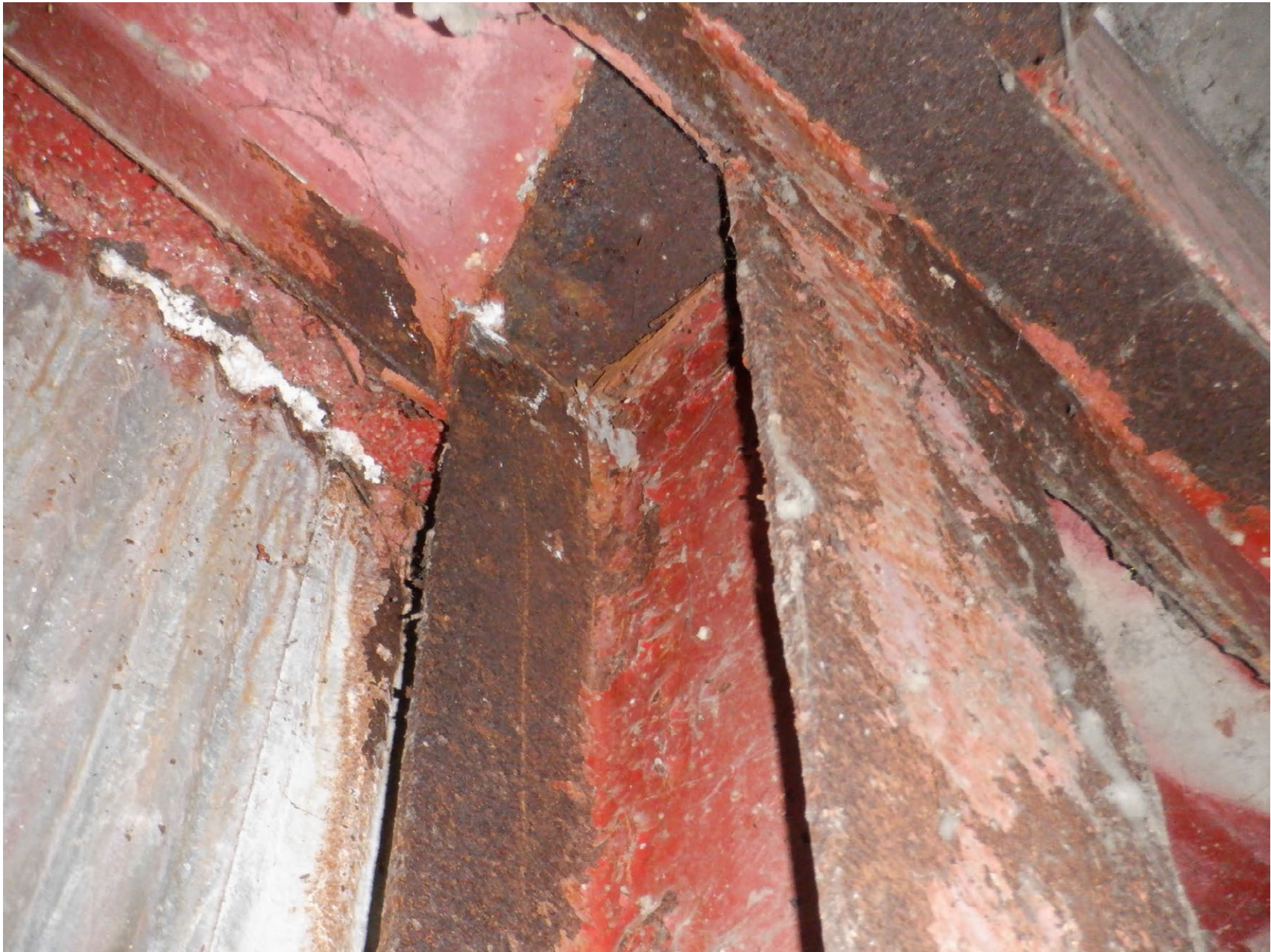
CORROSION AT TOP OF SOUTH ABUTMENT PILE 5W
