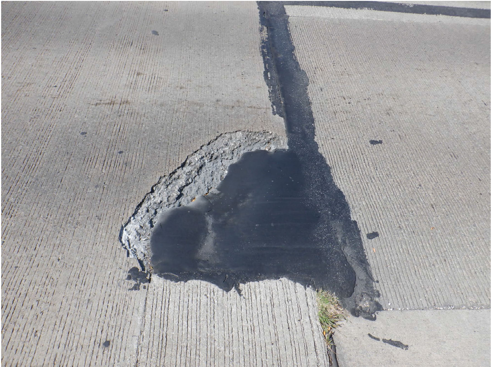
SPALL AT NORTH END OF DECK IN OUTSIDE NORTHBOUND LANE PARTIALLY FILLED WITH HOT-POURED RUBBER
