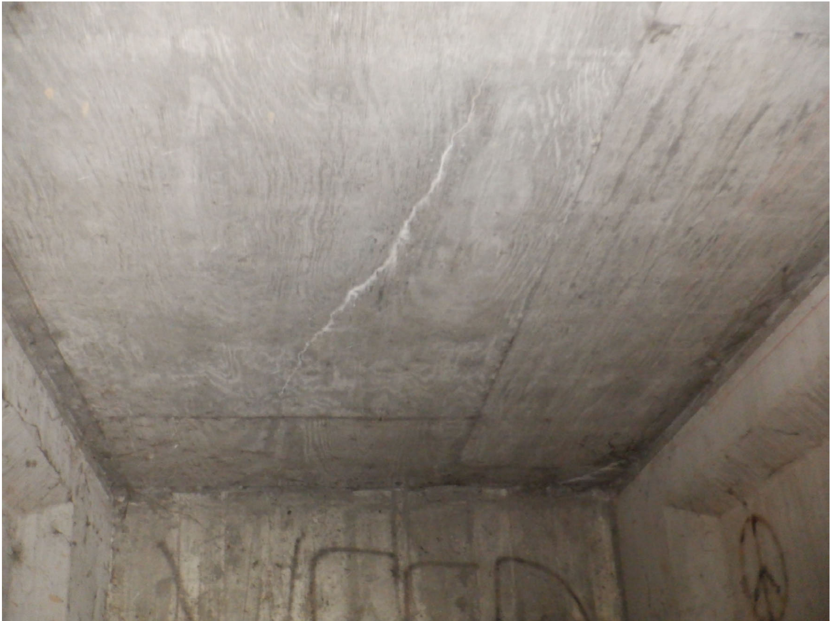
HAIRLINE LONGITUDINAL CRACKS WITH EFFLORESCENCE IN BOTTOM OF DECK AT EAST END
