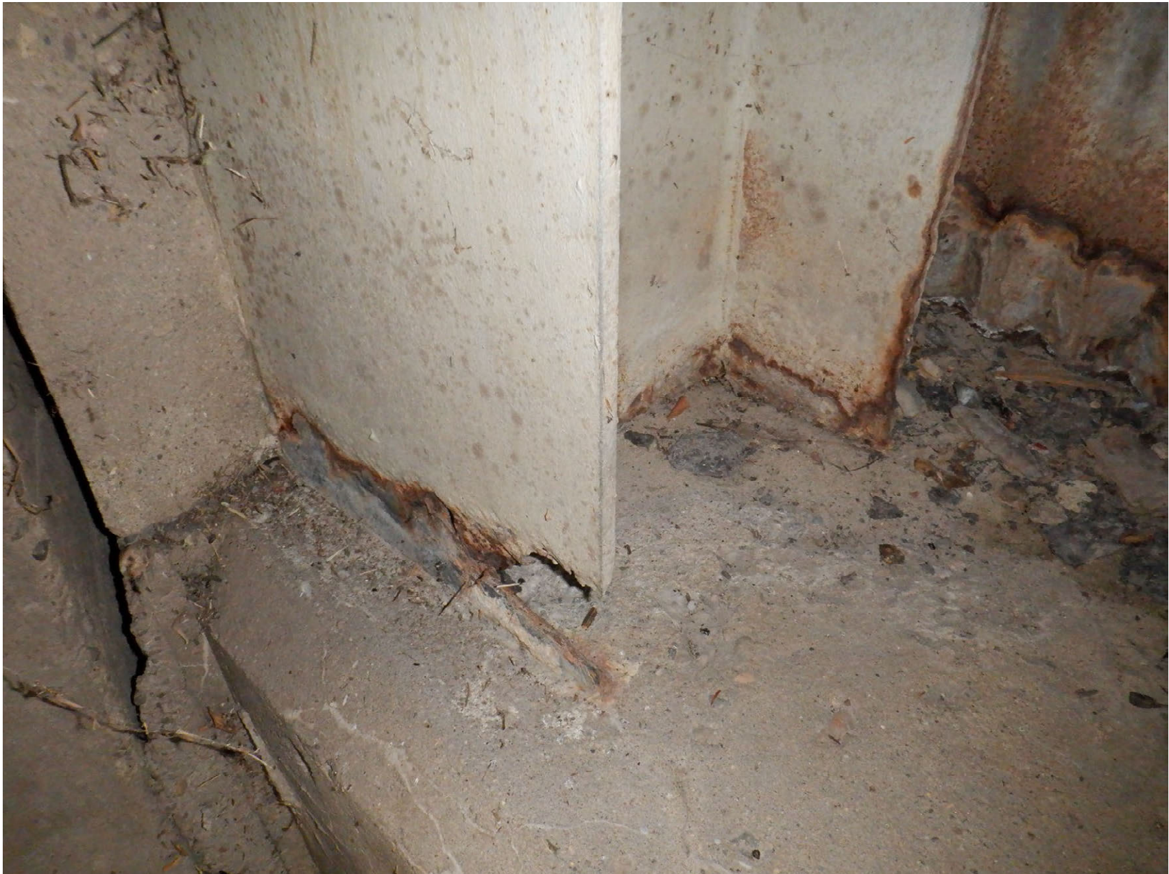
HOLE IN FLANGE OF NORTH ABUTMENT PILE UNDER WEST FASCIA
