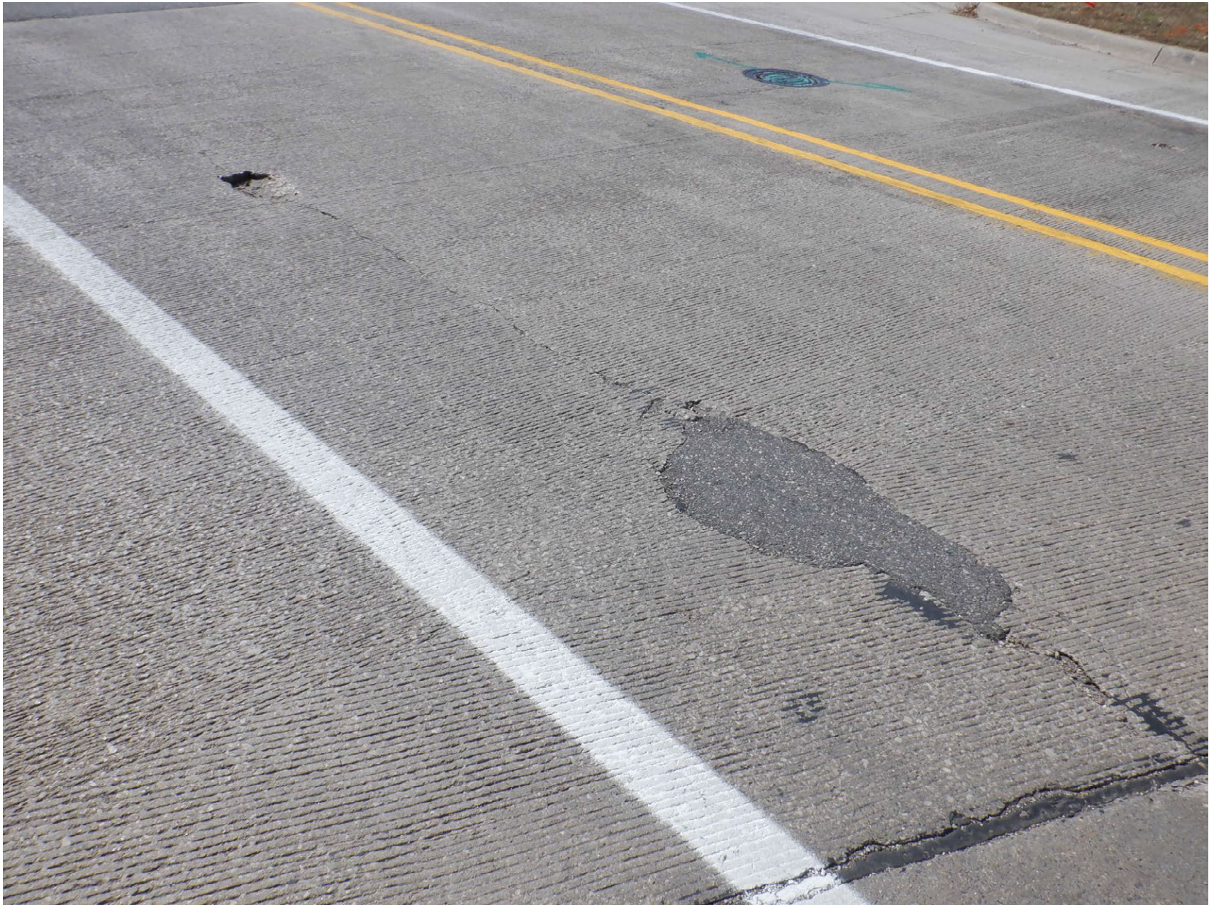
LONGITUDINAL CRACK AND SPALLS IN SOUTH APPROACH SLAB
