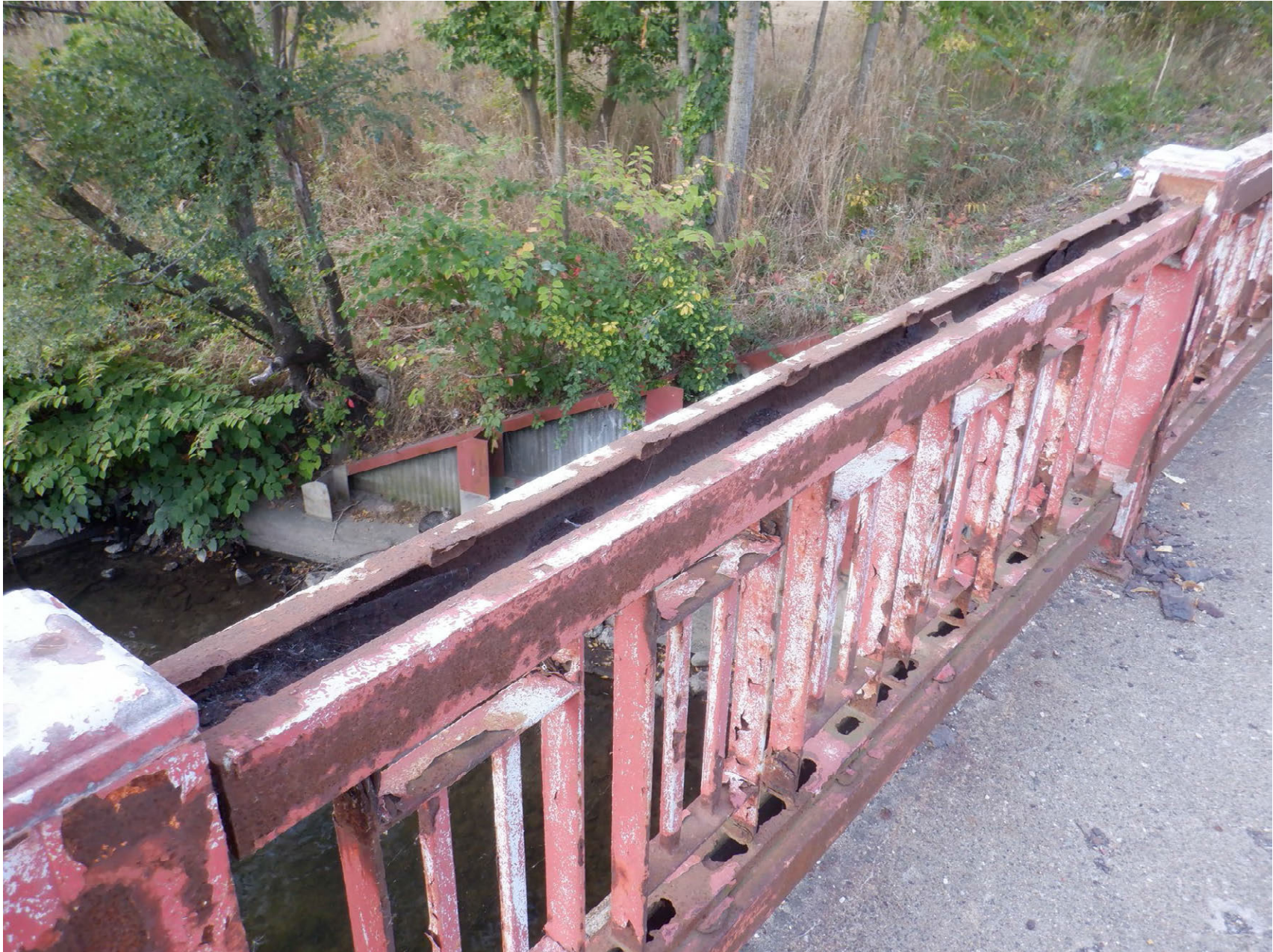
TOP RAIL PLATE MISSING EAST SIDE
