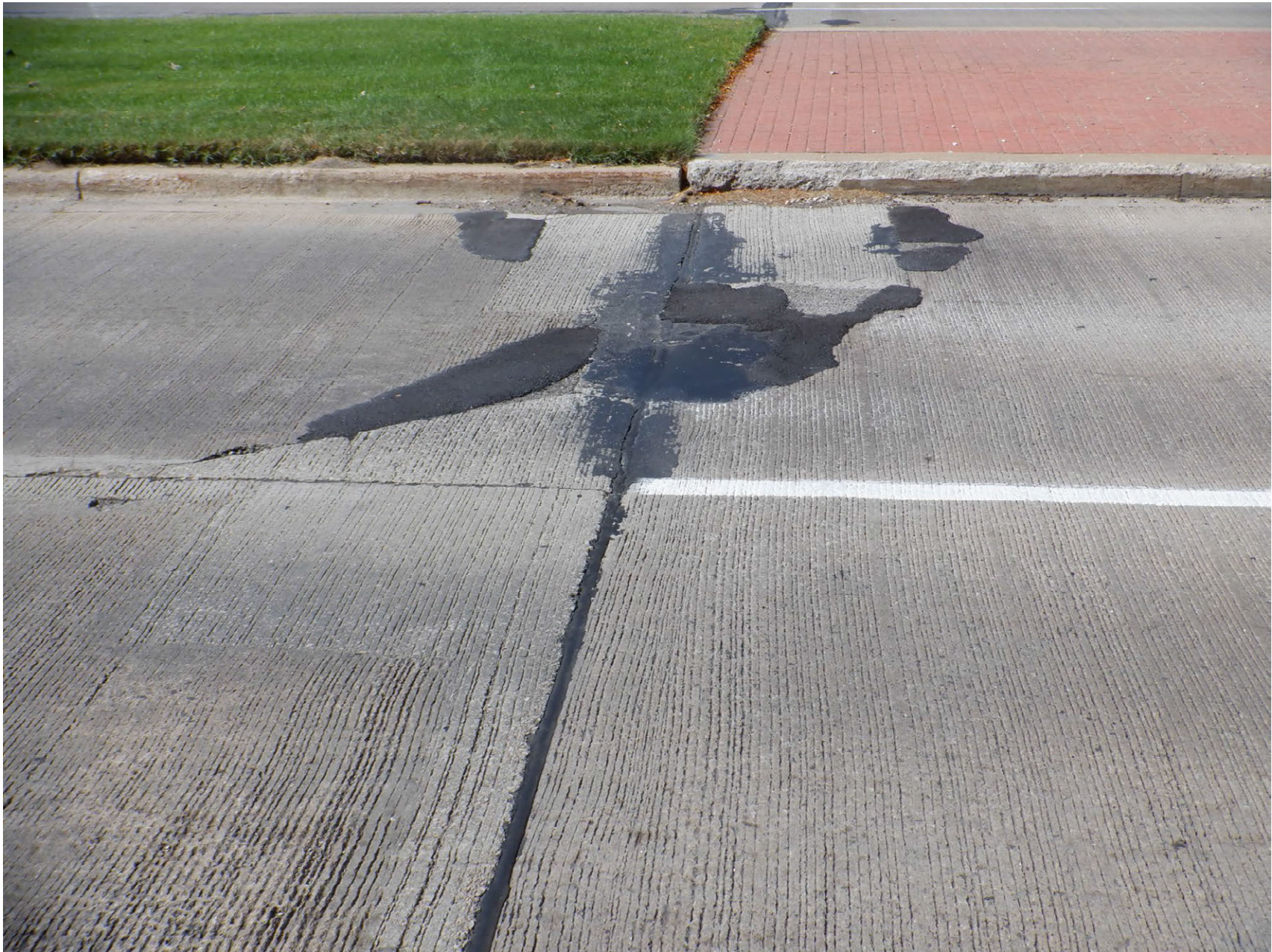
PATCHED SPALL AT SOUTH END OF DECK, INSIDE NORTHBOUND LANE
