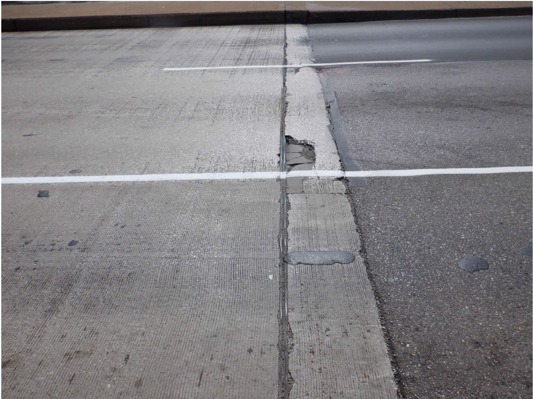
TOP OF BACKWALL SPALLED AT WEST END IN WESTBOUND LANE, JOINT FULL OF DIRT
