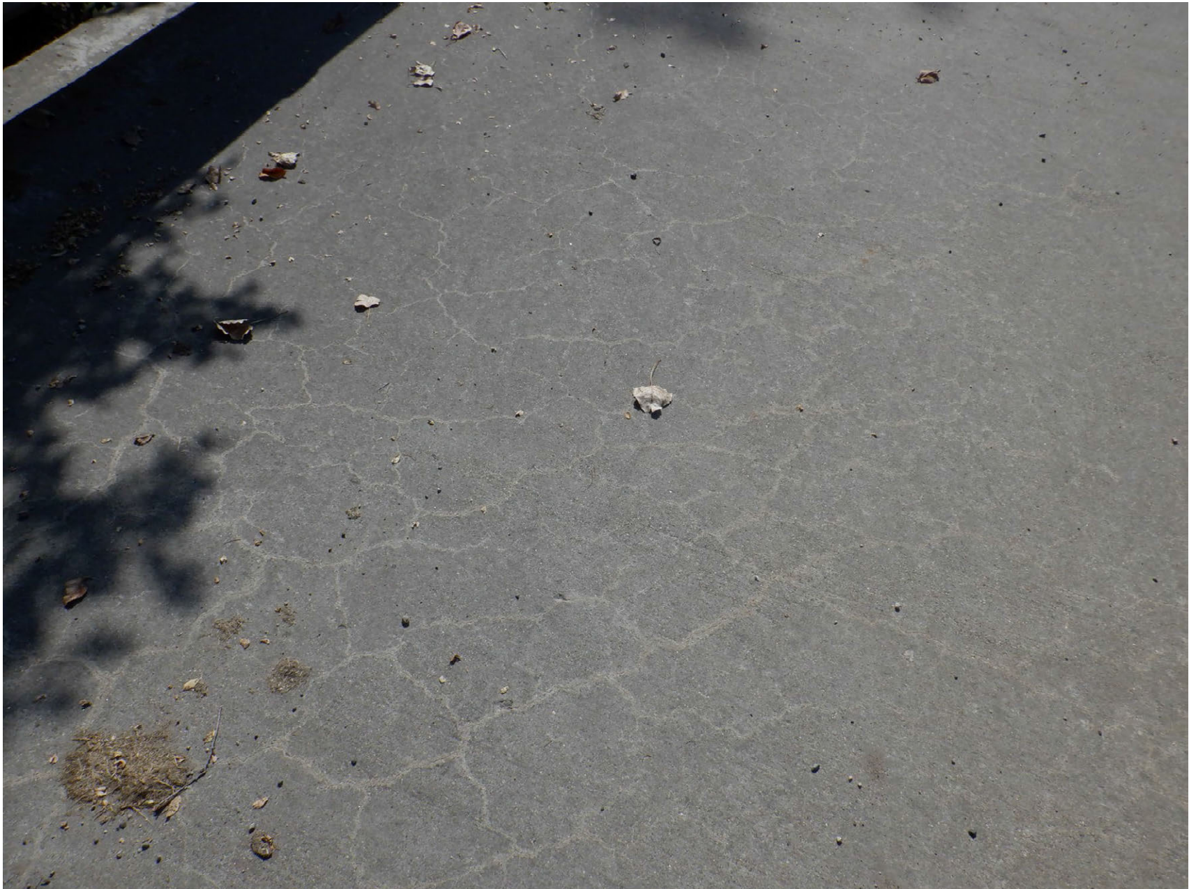
HAIRLINE SHRINKAGE CRACKING IN CONCRETE SIDEWALK
