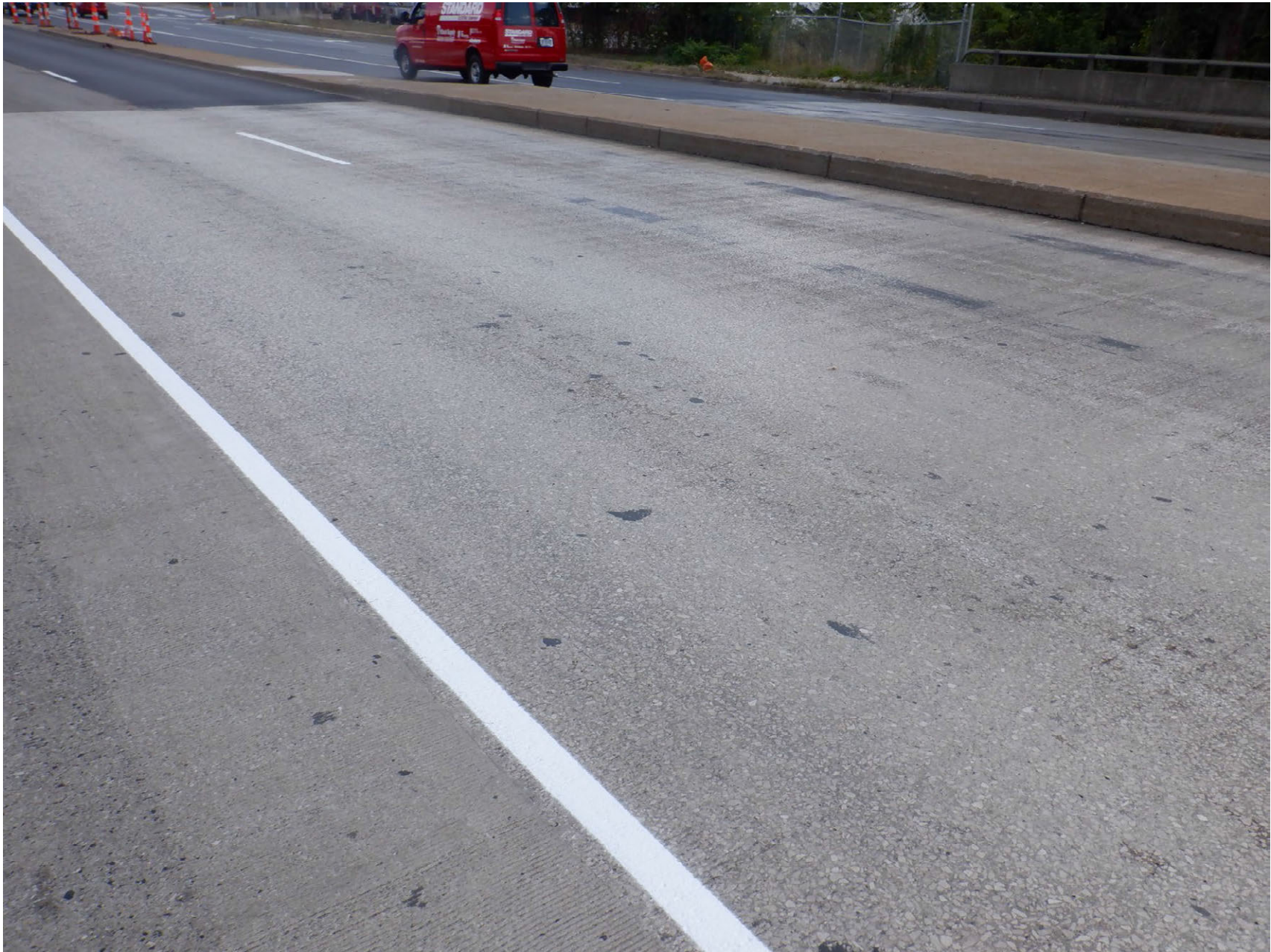
ABRASION OF CONCRETE DECK SURFACE IN TRAVEL LANES
