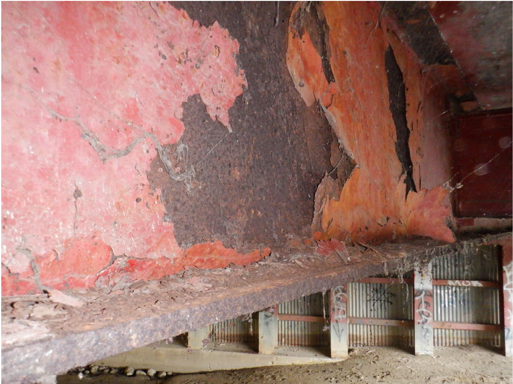
SECTION LOSS ON BOTTOM FLANGE AND WEB OF BEAM 4E AT MIDSPAN
