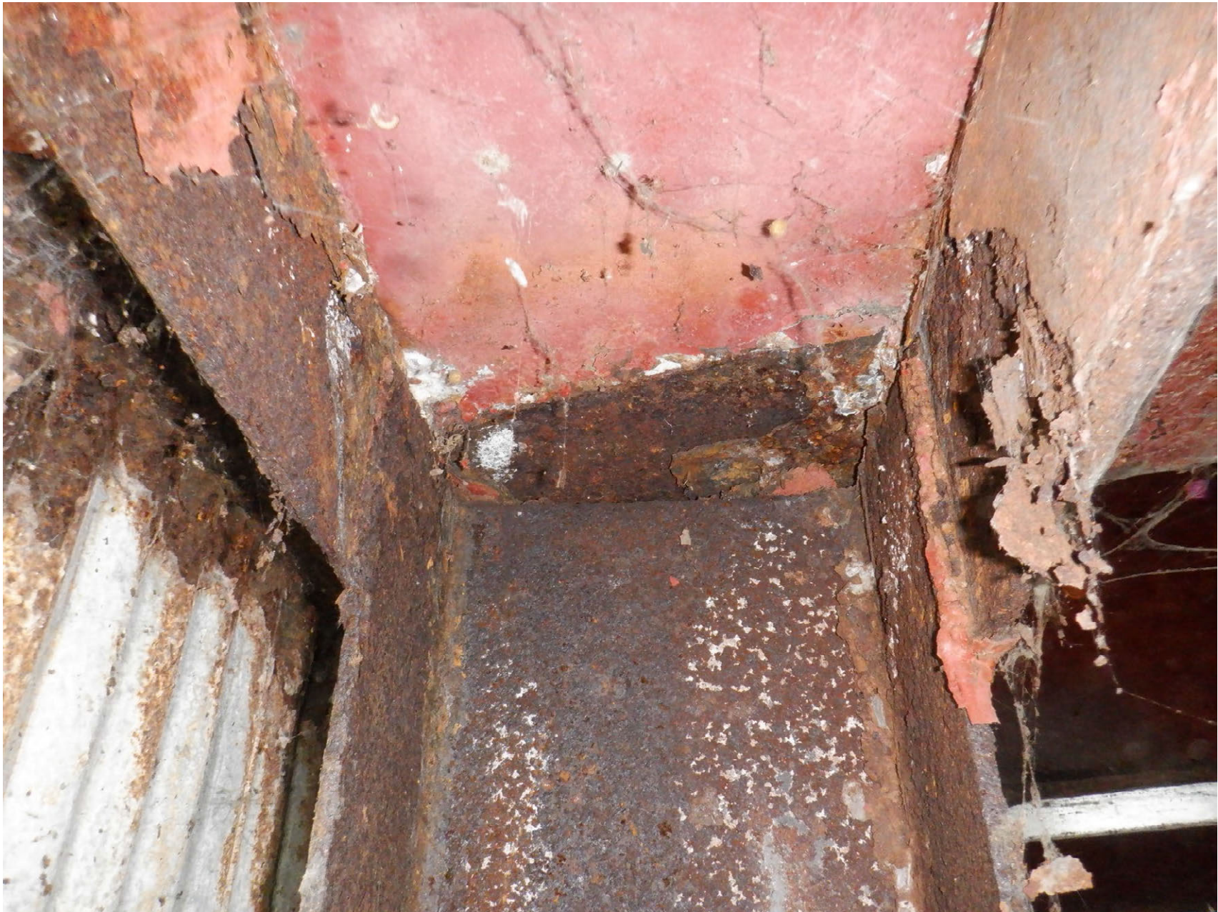
CORROSION/SECTION LOSS AT TOP OF NORTH ABUTMENT PILE 5W
