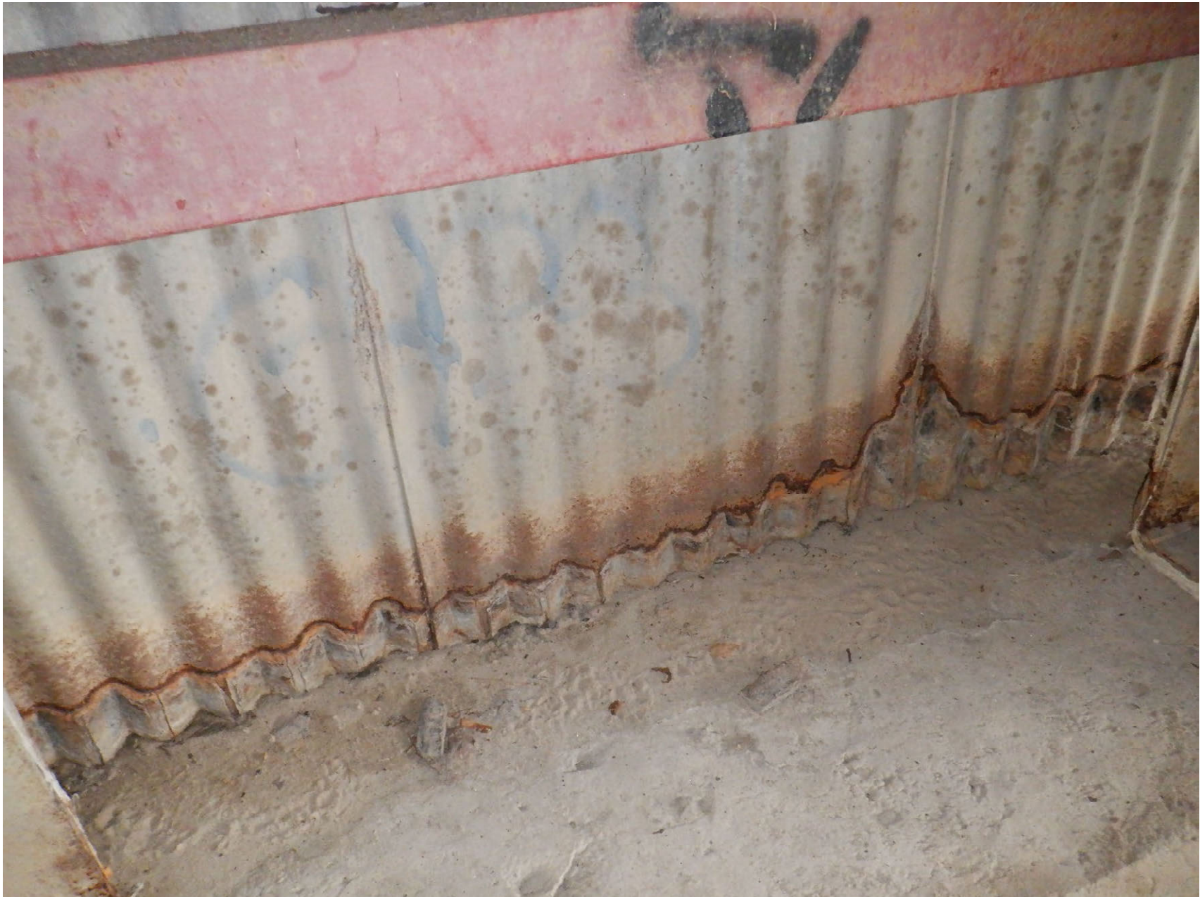
CORROSION ALONG BOTTOM OF CORRUGATED STEEL BACKWALL
