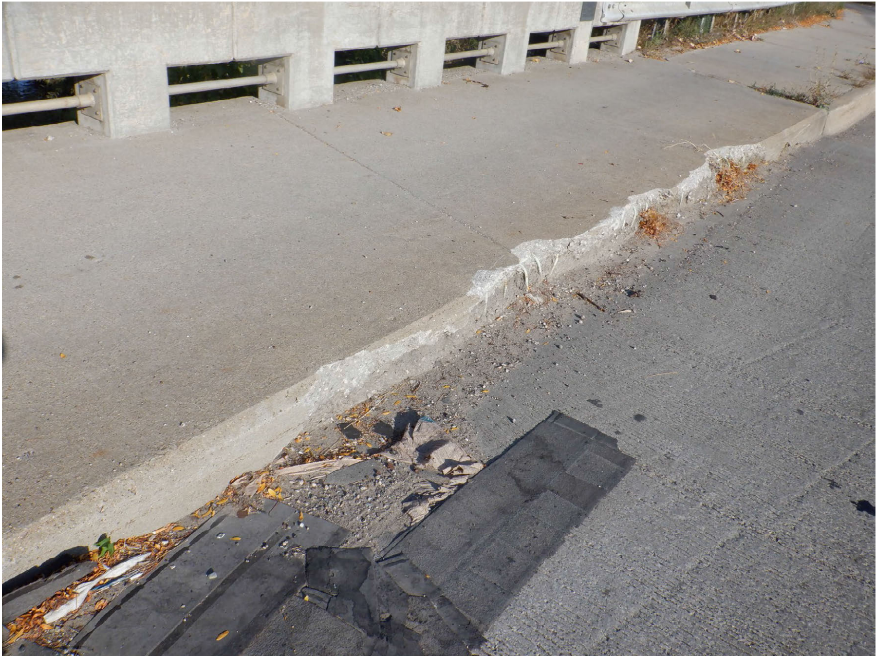
SPALLING WITH EXPOSED REBAR ALONG TRAFFIC FACE OF WEST SIDEWALK AT NORTH END
