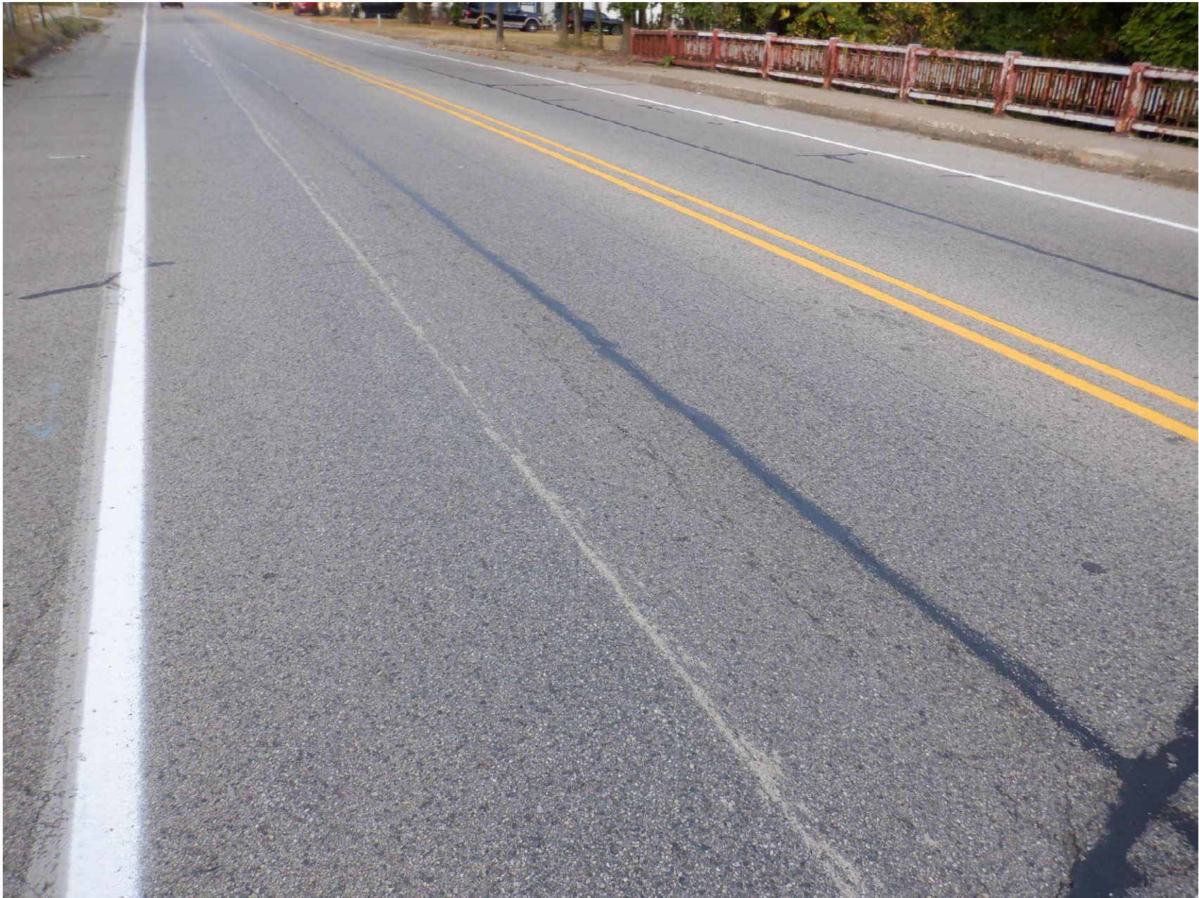
SEALED LONGITUDINAL CRACKS AND A FEW UNSEALED CRACKS IN HMA SURFACE OVER BRIDGE
