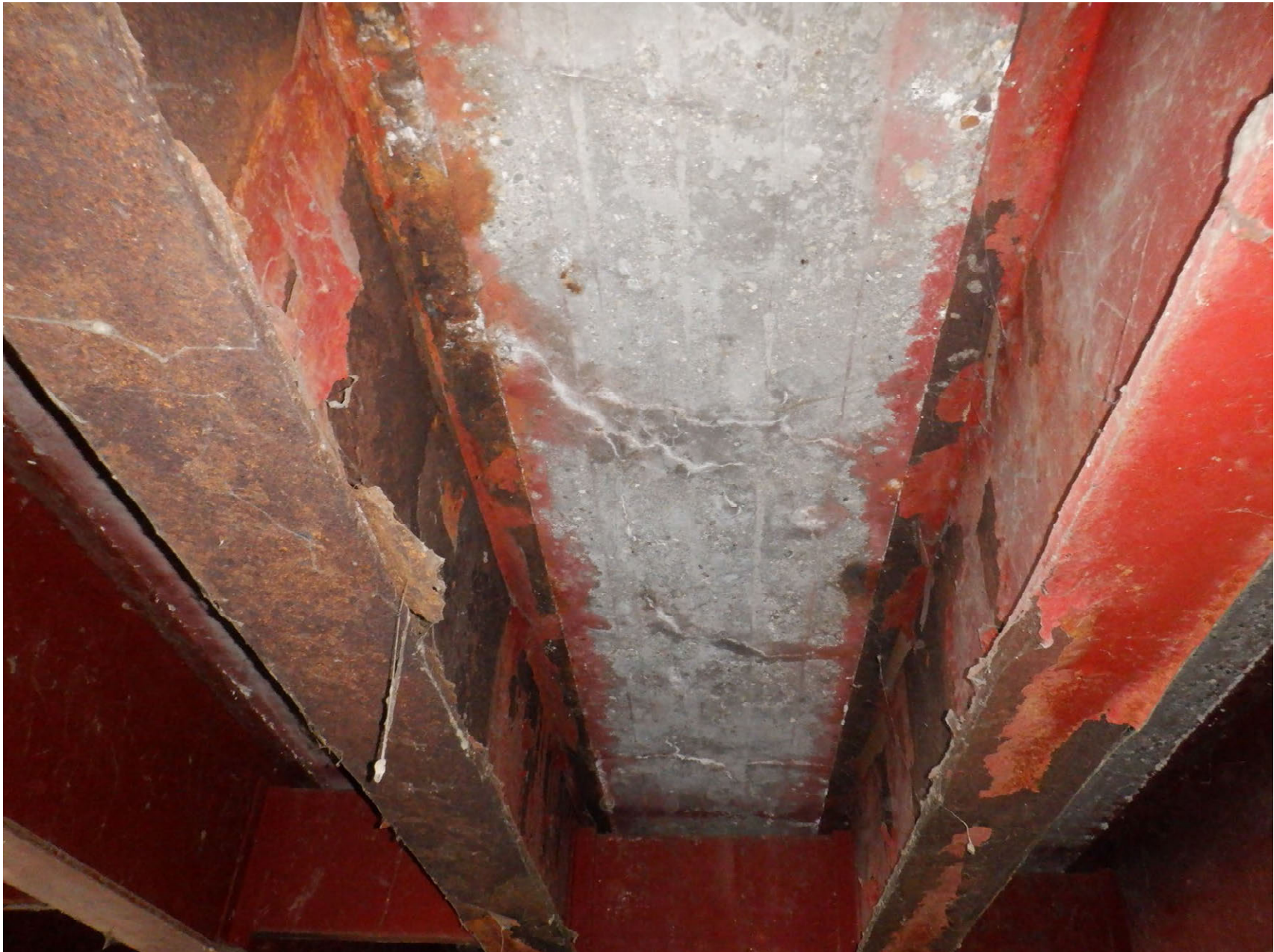
CRACKING WITH EFFLORESCENCE IN BOTTOM OF DECK
