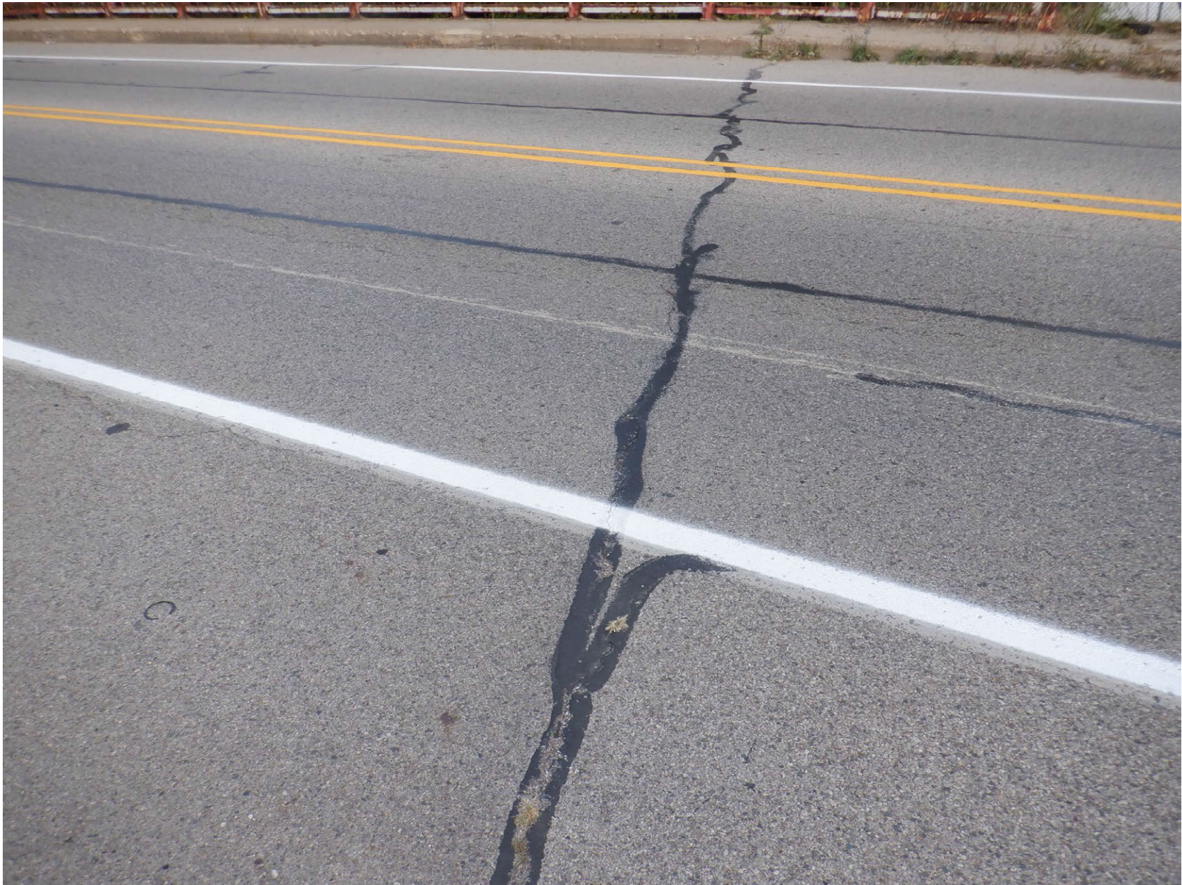
PARTIALLY SEALED CRACK IN HMA SURFACE AT NORTH REFERENCE LINE
