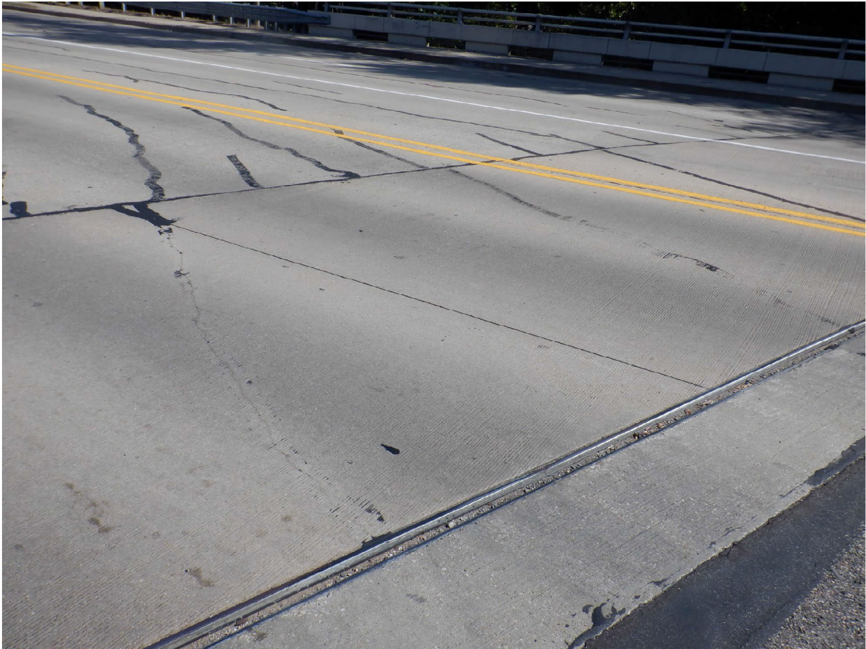
CRACKS IN SOUTH APPROACH SLAB PERPENDICULAR TO JOINTS, SOME PREVIOUSLY SEALED
