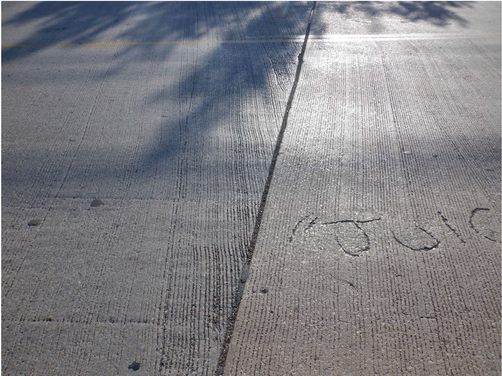
SEALANT MISSING AT SOUTH REFERENCE LINE JOINT, FULL OF DIRT
