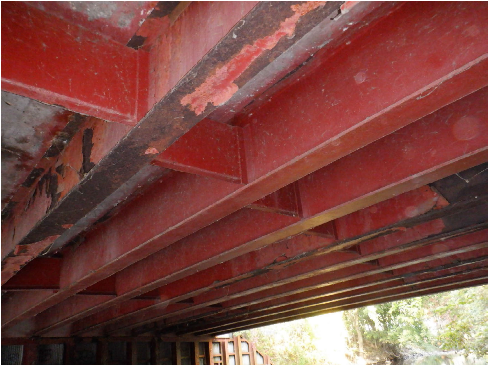
AREAS OF PEELING PAINT AND CORROSION ON STEEL BEAMS
