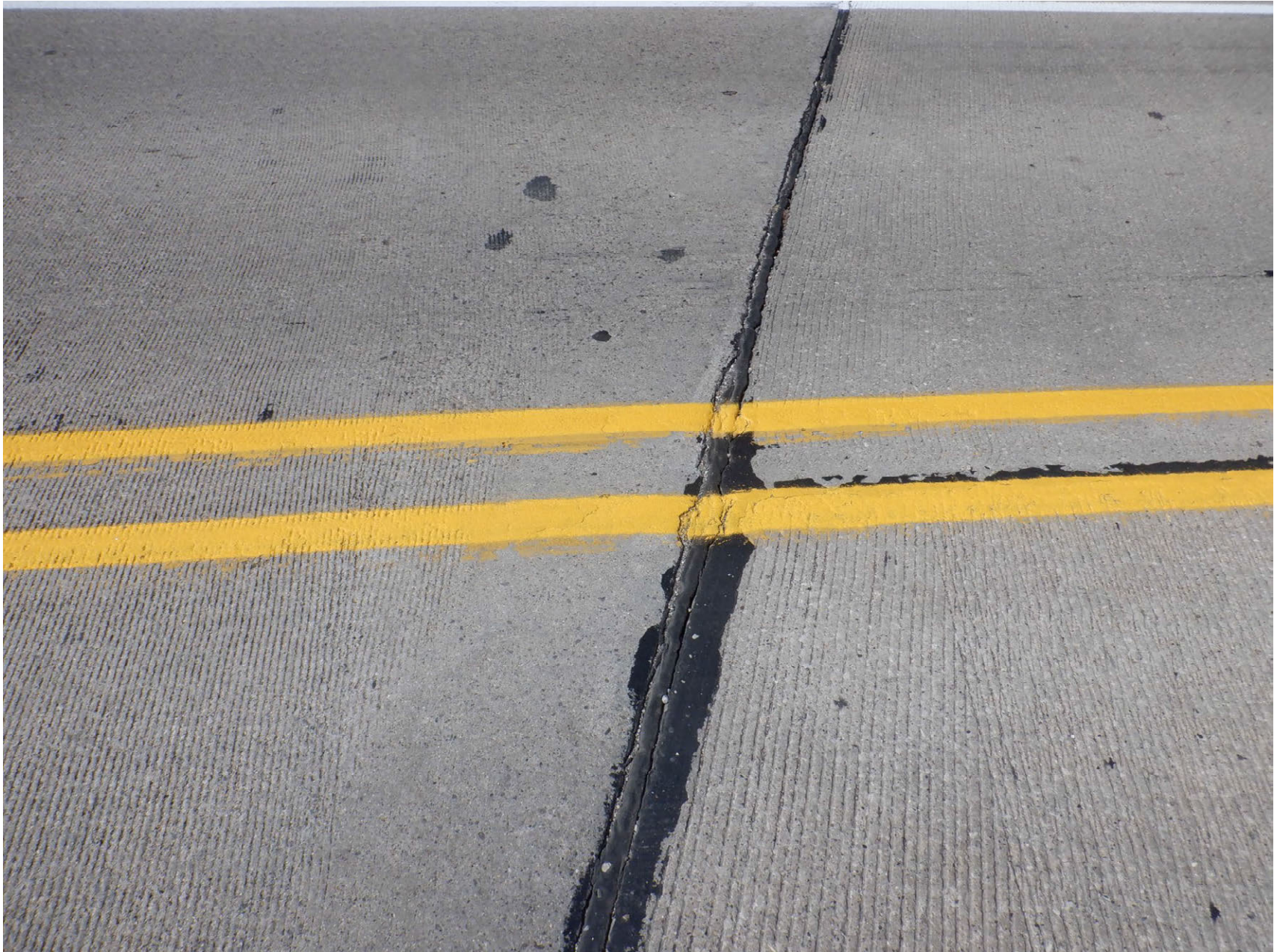
E3 JOINT SEALANT PULLING AWAY FROM CONCRETE AT NORTH REFERENCE LINE
