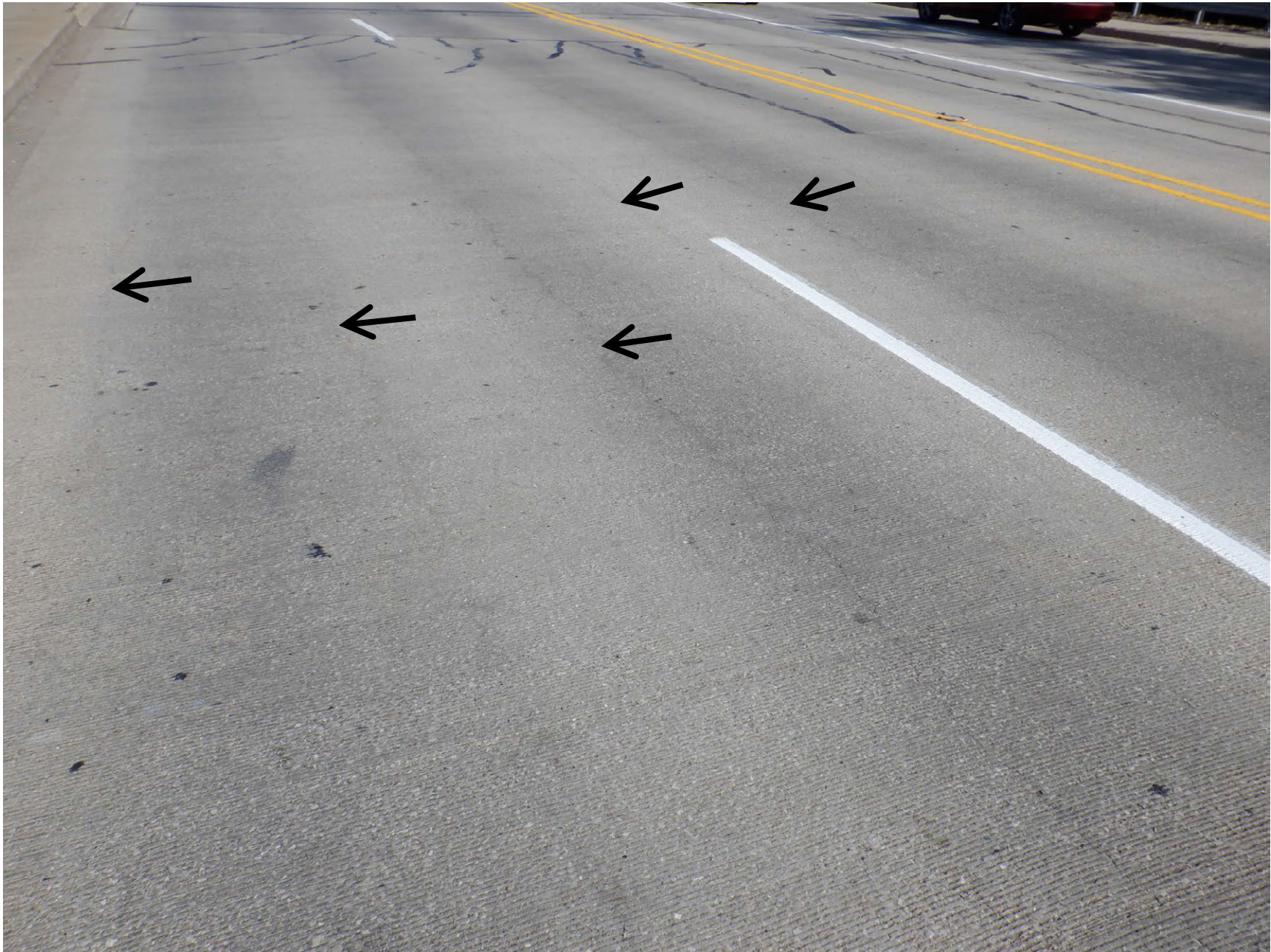
HAIRLINE LONGITUDINAL CRACKS IN CONCRETE DECK ALONG BEAM LINES
