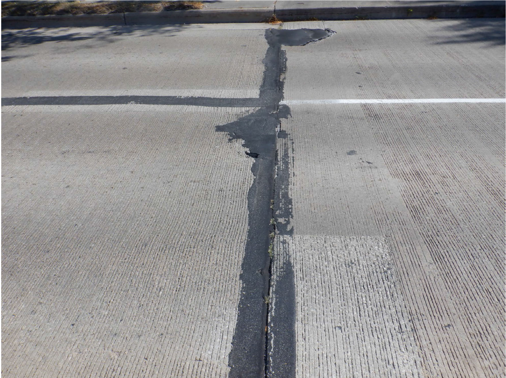
SEALANT AND PATCHING AT NORTH REFERENCE LINE
