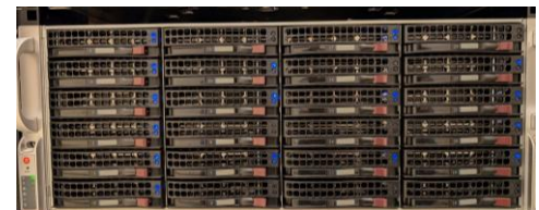
6-Year-Old Backup Server
