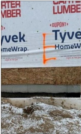
Meter location marked.
