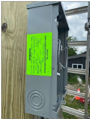
Meter socket inspection sticker.
